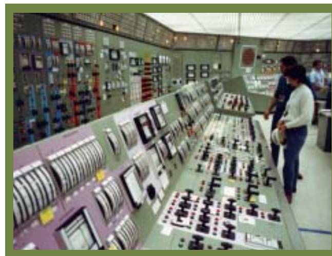
Nuclear power plant control room.
