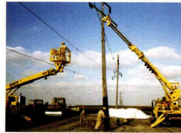
Corn Belt Power transmission crews modify a line to prepare for construction at Drager Switching Station near Glidden.
