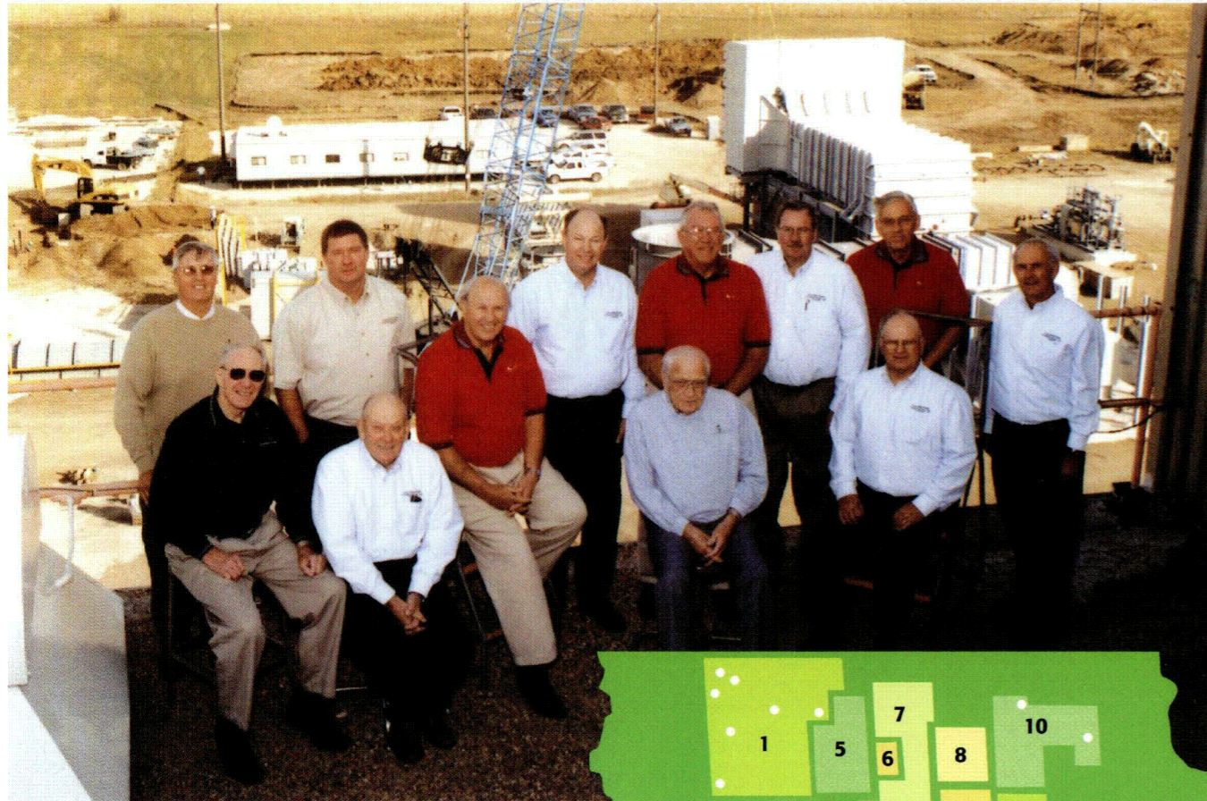
On the roof level of Wisdom Unit 1, overlooking Wisdom Unit 2 construction, are, front from left: John Schumacher, Glidden REC; Donald O'Tool, assistant secretary/treasurer, Calhoun County REC; Ronald Deiber, vice president, NIMECA; Roger Rust, Franklin REC; and Norman Kolbe, Sac County REC. Second row from left: Donald Feldman, president, Butler County REC; Scott Stecher, Prairie Energy Cooperative; Charles Gilbert, treasurer, Midland Power Cooperative; L. Kirby Range, Iowa Lakes Electric Cooperative; Donald McLean, secretary, Grundy County REC; LeRoy Weber, Humboldt County REC; and Dale Arends, executive vice president and general manager.
