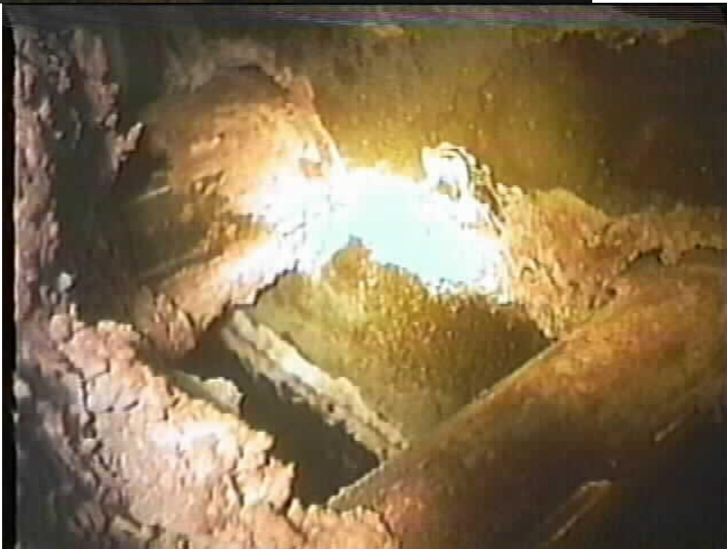
Figure 30. Flange Leakage Crusted On Side of Nozzles and Stalactites from Gaps in Insulation (8RFO)
