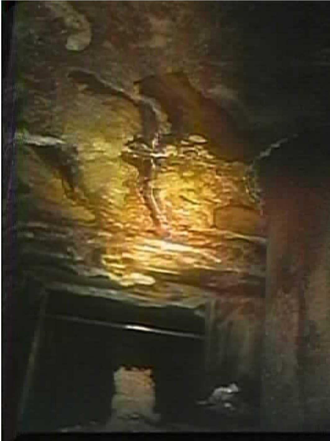
Figure 29. Flange Leakage with Stalactite Formation from Insulation and Stalagmite Formation on top of Reactor Vessel Head (8RFO)
