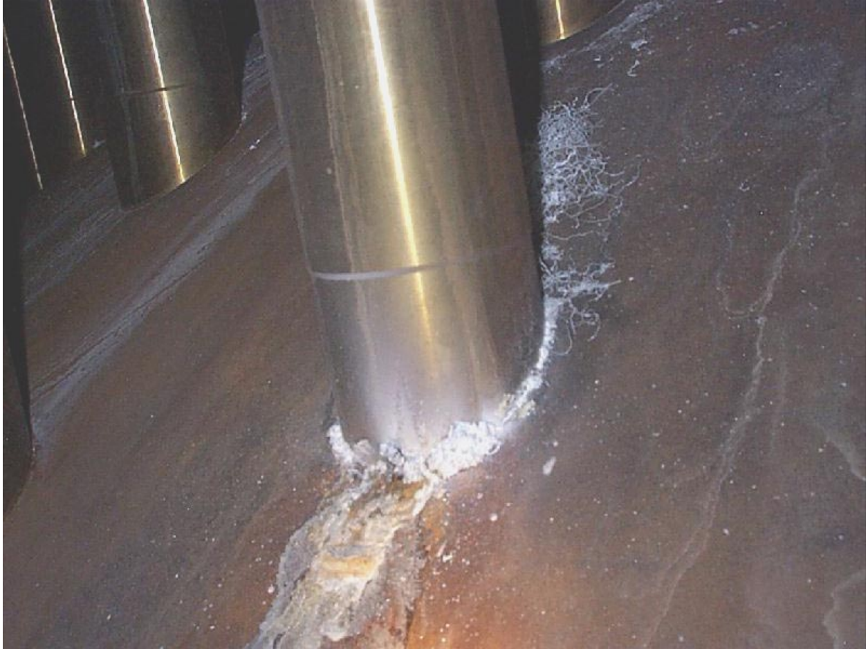
Figure 18. CRDM Nozzle Leakage Observed at Oconee 3
