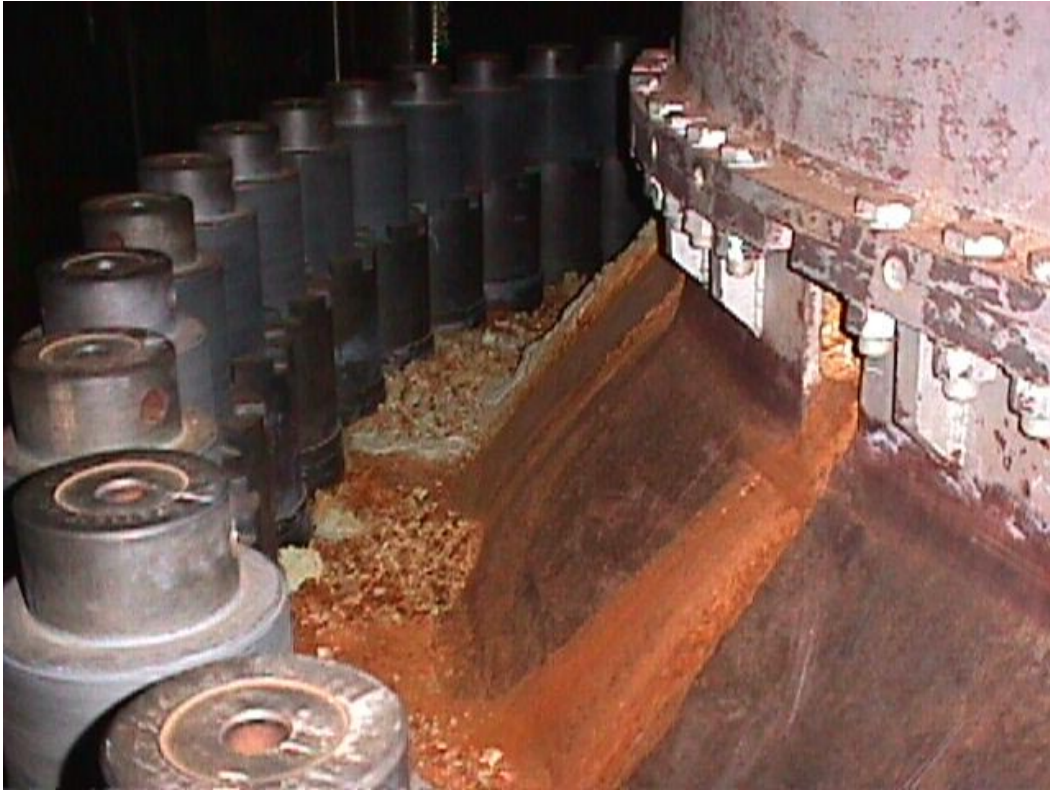
Figure 4. Boric Acid and Iron Oxide on Vessel Flange at 12RFO
