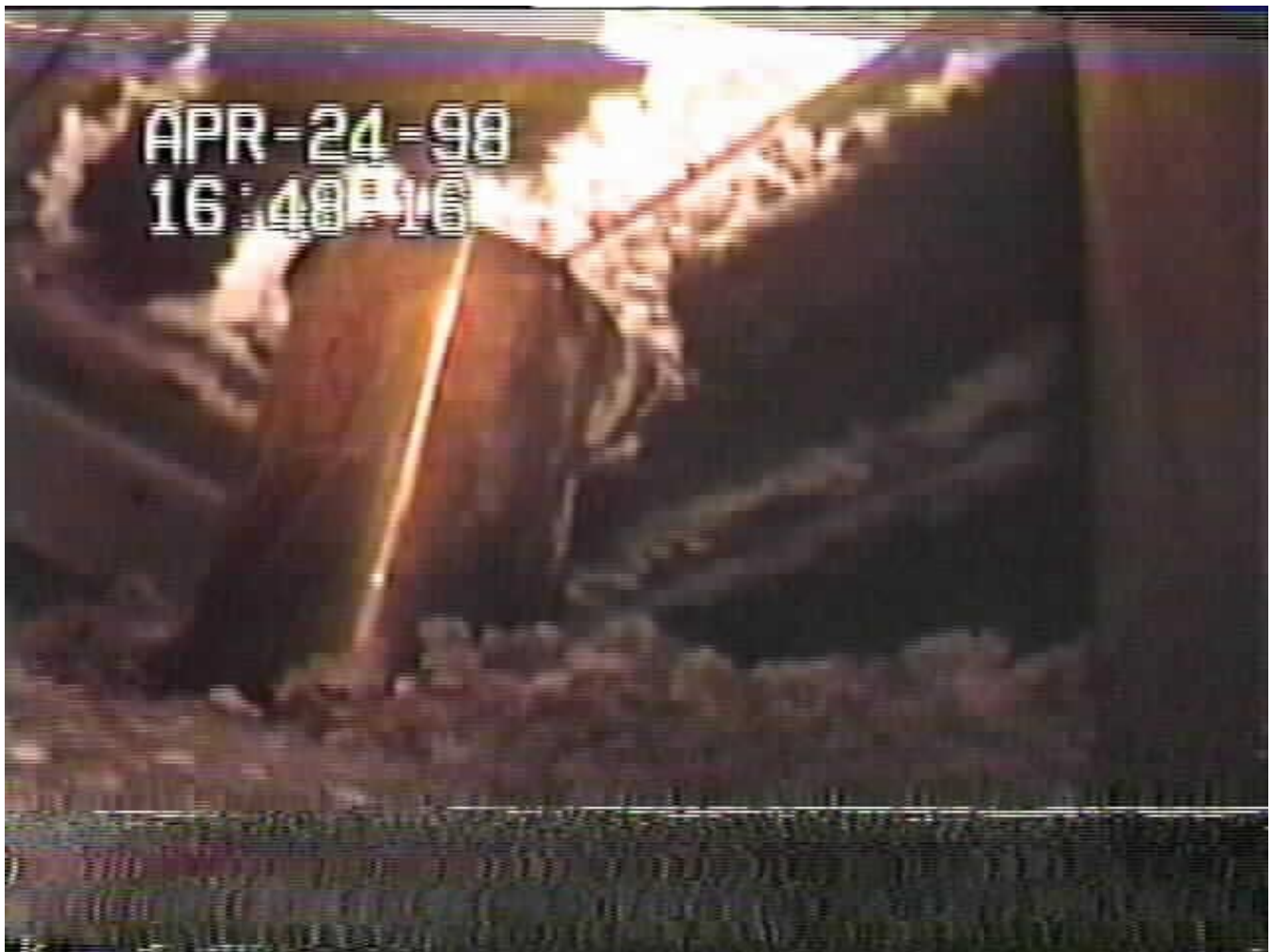
Figure 37. Boron Piled Under the Insulation (11RFO)
