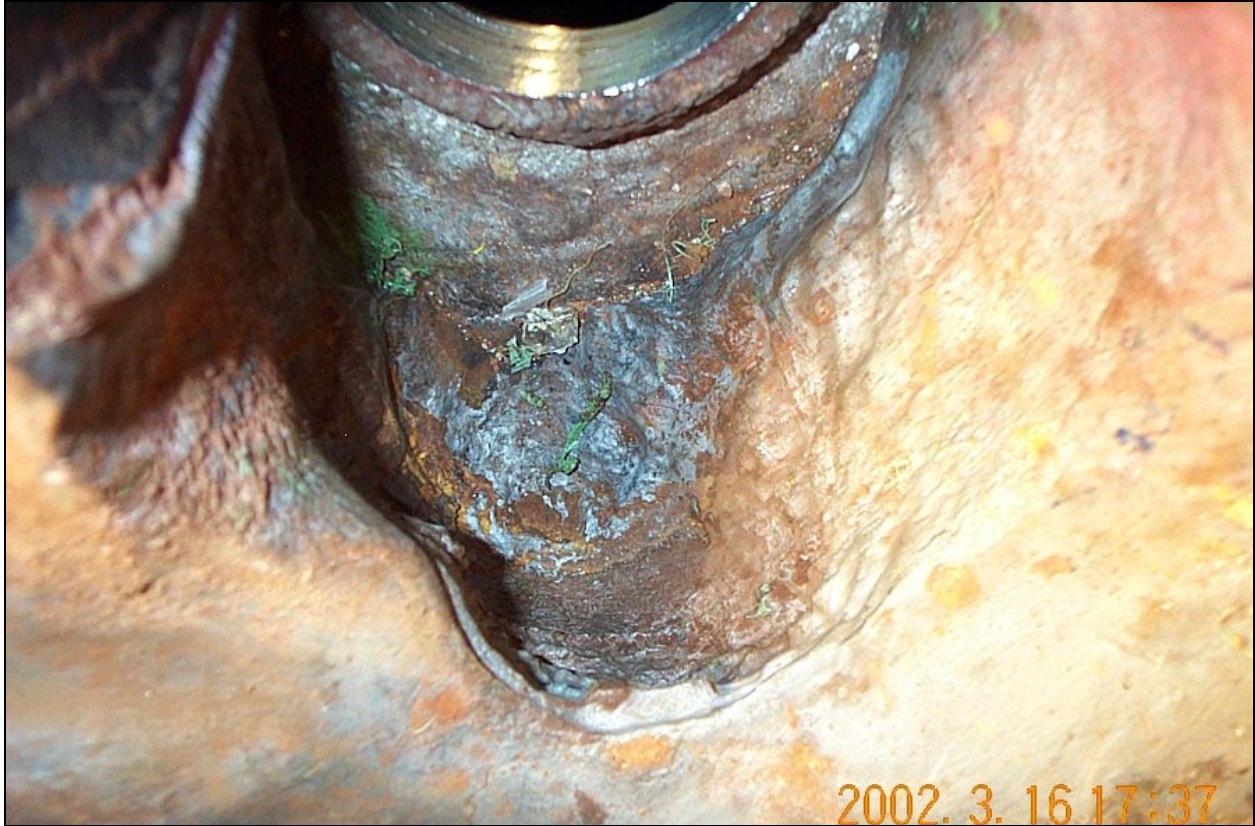
Figure 6. Cavity in Reactor Vessel Head Between Nozzle 3 and 11
