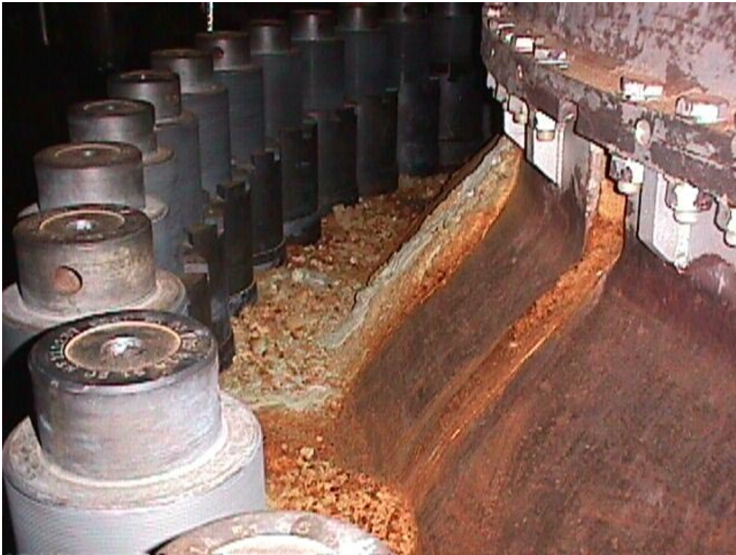
Figure 36. Red Rusty Boric Acid Deposits on Vessel Flange at 12RFO
