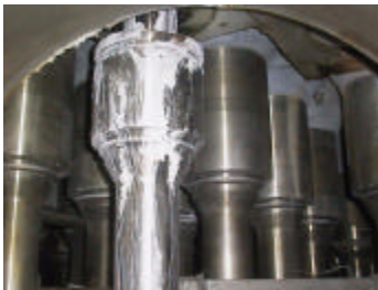
Figure 11 - CRDMP No. 75 L-15 Conoseal Leakage Path at CRDM Column (As Found)
