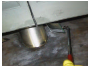
Figure 16 - CRDMP No. 75 L-15 Conoseal/CRDM Column at Penetration to RPV Head Interface ( After cleaning )
