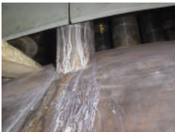
Figure 15 - CRDMP No. 75 L-15 Conoseal Leakage Path at Penetration to RPV Head Interface ( As Found )
