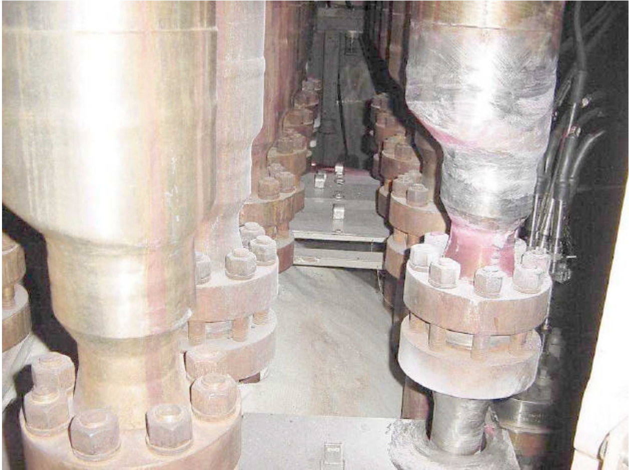
Palisades Plant Reactor Pressure Vessel Head with Some Insulation Access Panels Removed
