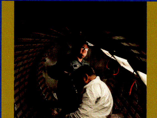
Hundreds of specialized outside contractors, along with Alliant Energy employees, performed extensive work at six power stations during early 2000 to ensure electric reliability during peak summer months.
