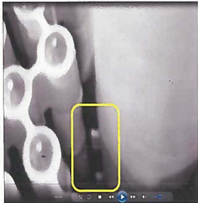
Figure 2: Closeup of Spacer 8 Water Rod Tab
