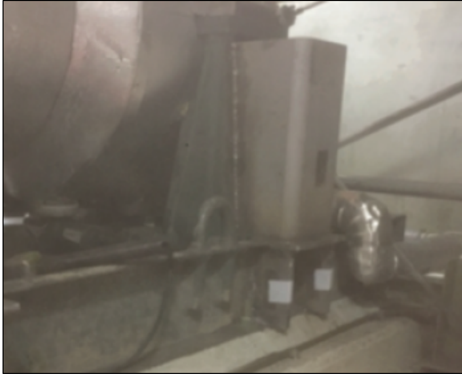
Figure 2: Post-Modification Photo of the 2MSIBP02 Pump Pedestal with Added Box Steel and Gussets
