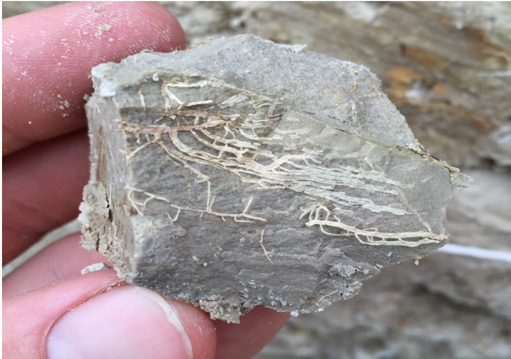
Figure 4-16 Small Roots Grow in Thin Structural Cracks in the Radon Barrier at Falls City TP-4 These cracks are common along the edges of clay clods that remain from construction. TP-4 was a control, located many meters from a mesquite bush.
