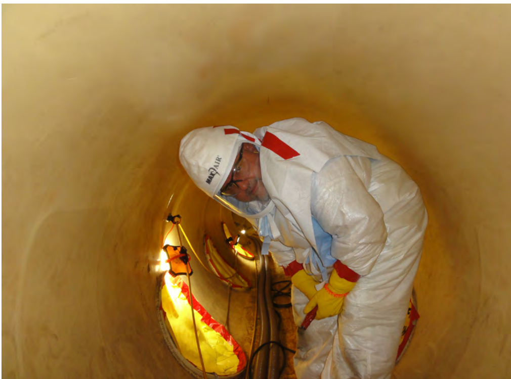
NRC resident inspector Thomas Taylor effectively oversees repairs of Fermi Nuclear Power Plant's torus during a refueling outage. The torus is a massive donut-shaped reservoir located below the reactor.
