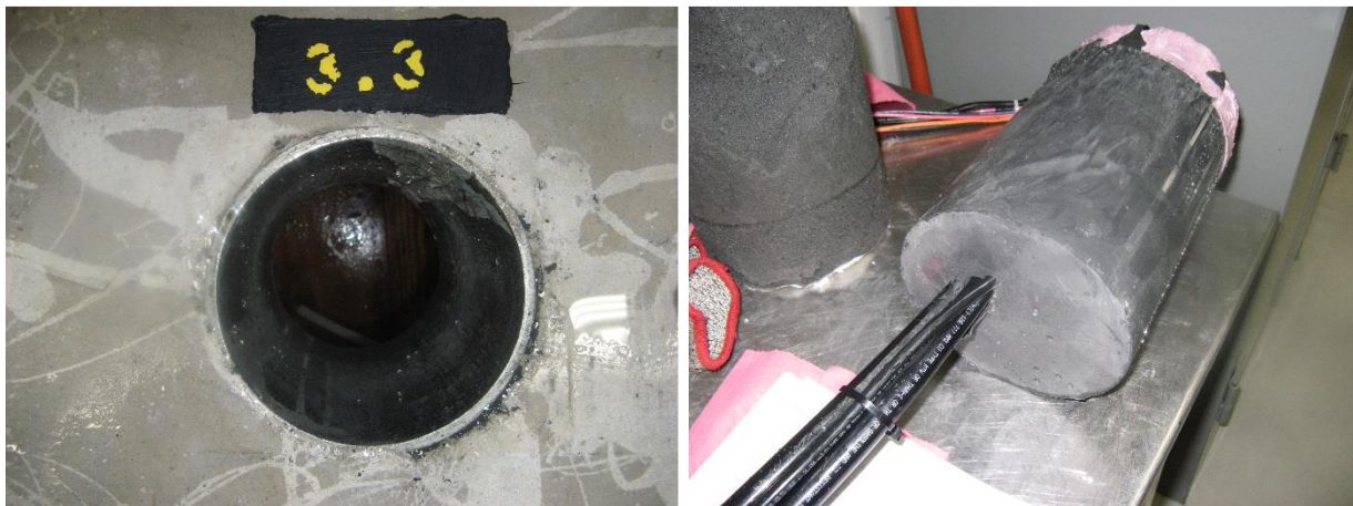
Figure 5-24 Empty Steel Sleeve for Ejected Penetration 3.3 (Left Photo) and Ejected Seal Material and Penetrants for Penetration 3.3 (Right Photo)
