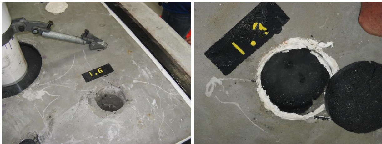
Figure 5-4 Empty Penetration 1.6 (Left Photo) and Damaged Penetration 1.3 (Right Photo)
