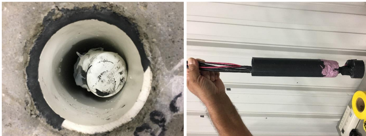
Figure 5-8 Top-Down View (Left Photo) of Penetration 2.2 Dislodged with its White Cable Cap Visible and Penetration 2.2 Removed (Right Photo) from the Test Deck (its White Cable Cap Not Visible)
