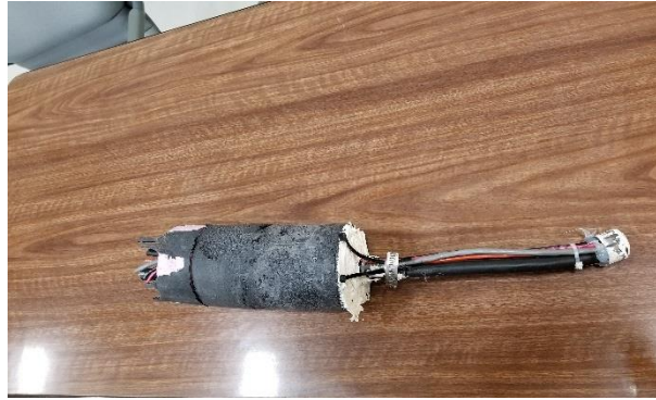
Figure 5-13 Ejected Seal and Penetrant from Penetration 2.6
