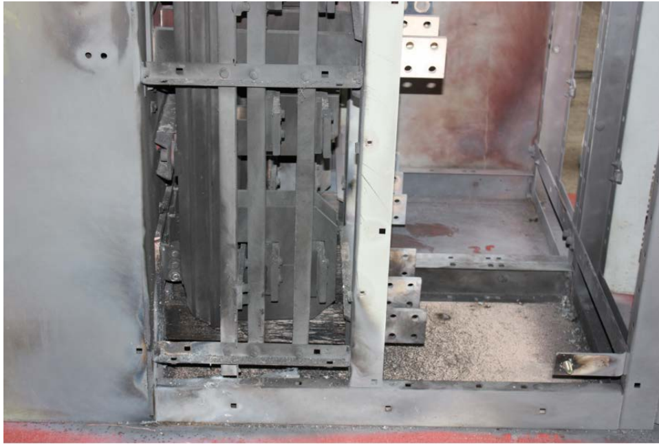
Fig. 63. Enclosure Post-Test 2-13G.
