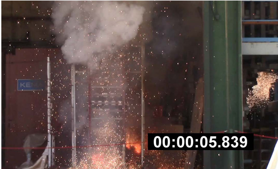
Fig. 76. Failure of KEMA cable connection observed as arcing occurring in Cell 8 (non-test cell).
