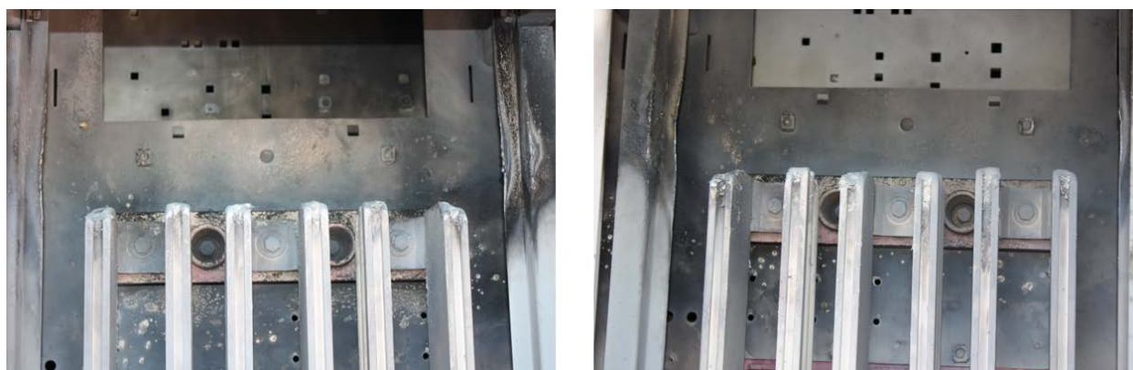
Fig. 68. Enclosure Post-Test 2-18A. Top of main bus, Load side (left), supply side (right).
