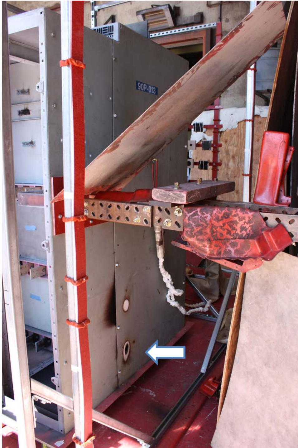
Fig. 69. Post-experiment image of enclosure breach and thermal effects on supply side of gear.
