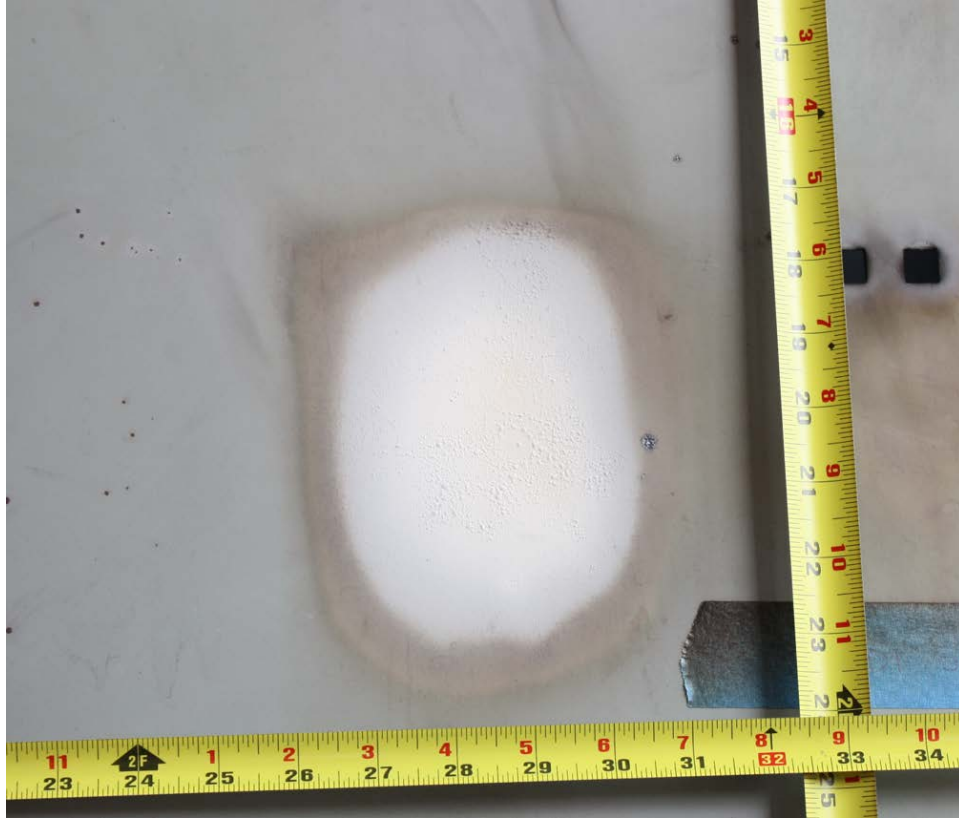
Fig. 47. Thermal heating on external of load section enclosure adjacent to top of vertical bus bars.
