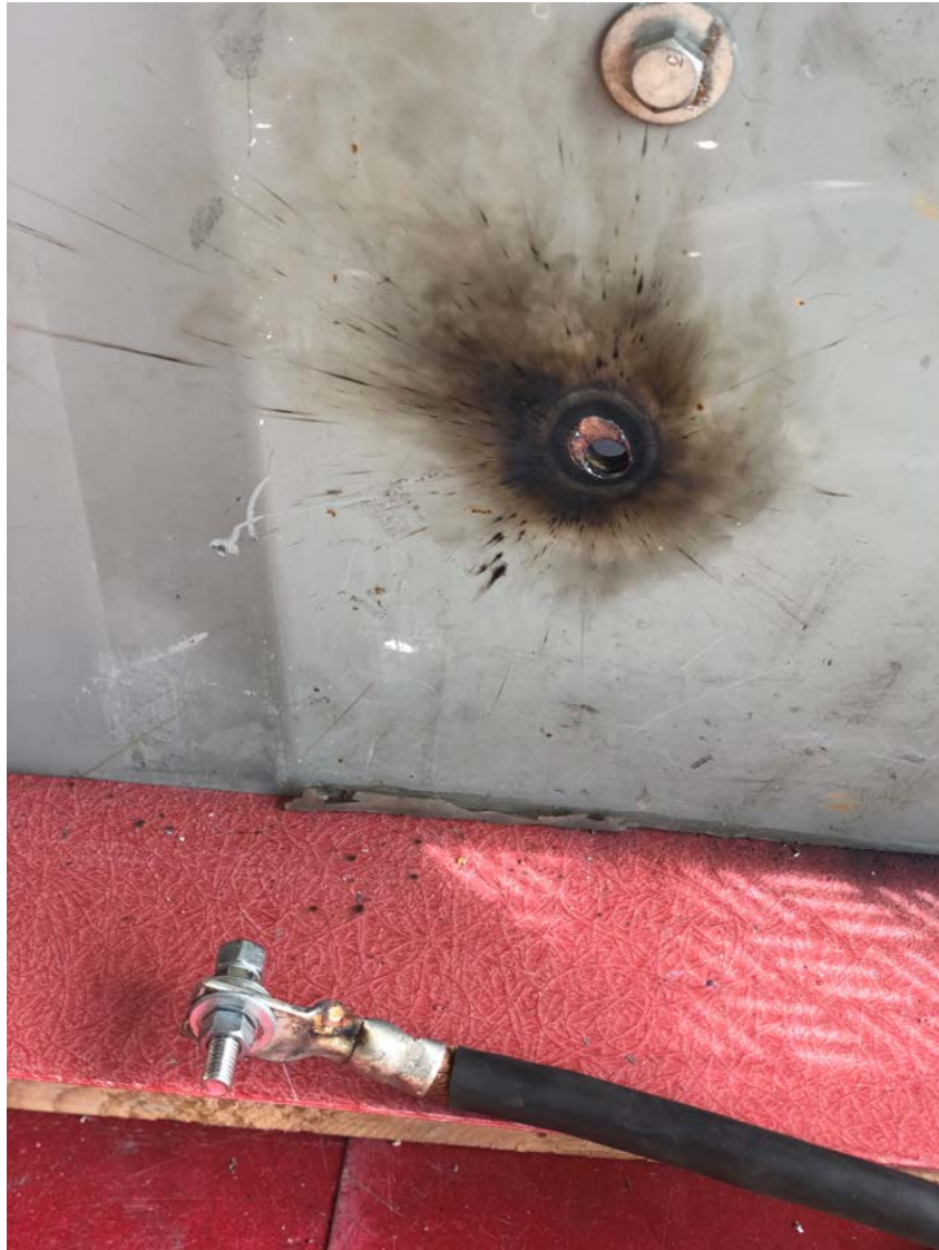
Fig. 59. Post-experiment image of enclosure grounding cable disconnected from enclosure due to current flow through ground circuit.
