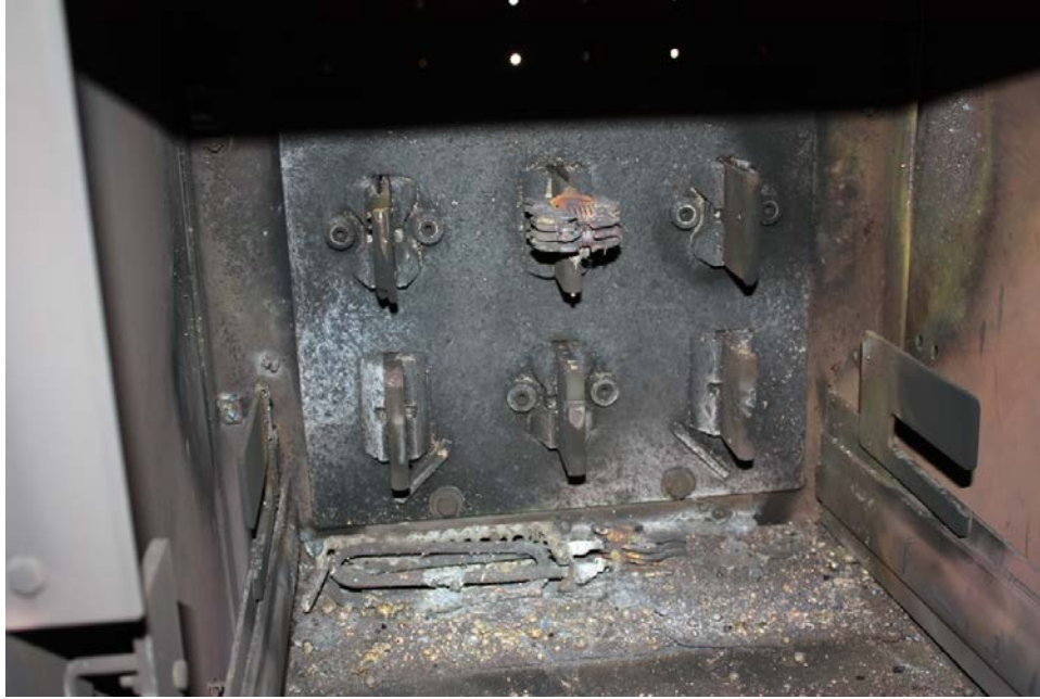
Fig. 52. Switchgear stabs post-experiment.
