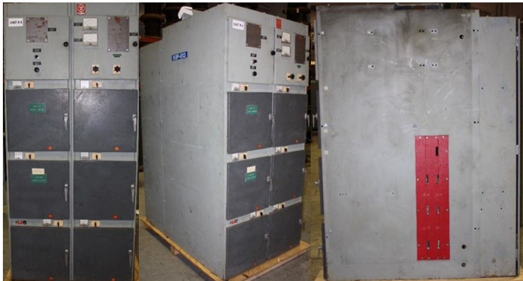
Fig. 5. Photo of DS switchgear. (front (left); side and front (center); opposite side (right)).
