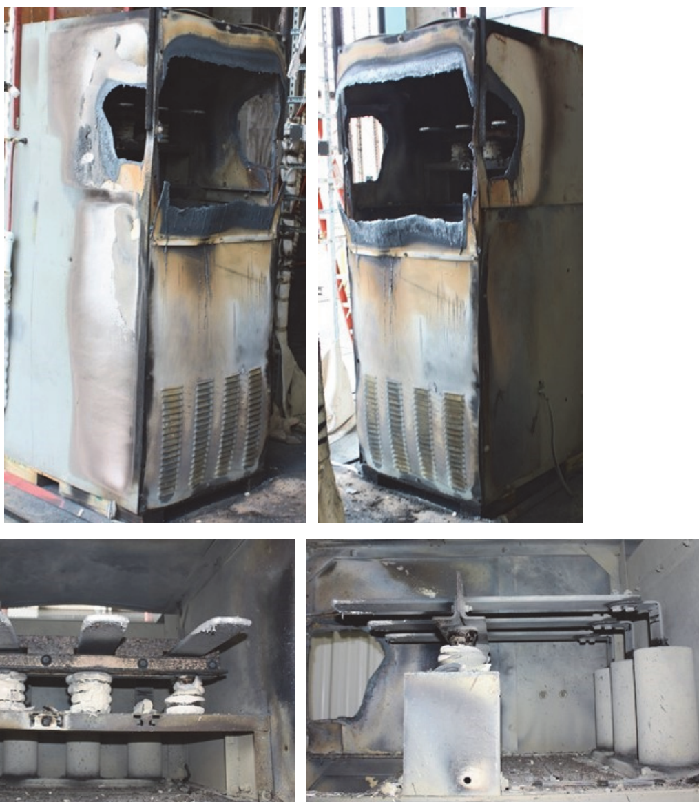
Fig. 79. Enclosure Post-Test 2-24. (Top: back of enclosure; Bottom: remaining bus bar material. Bottom left as viewed from rear of enclosure, bottom right as viewed from the side at the rear of the enclosure with the side panel removed.)
