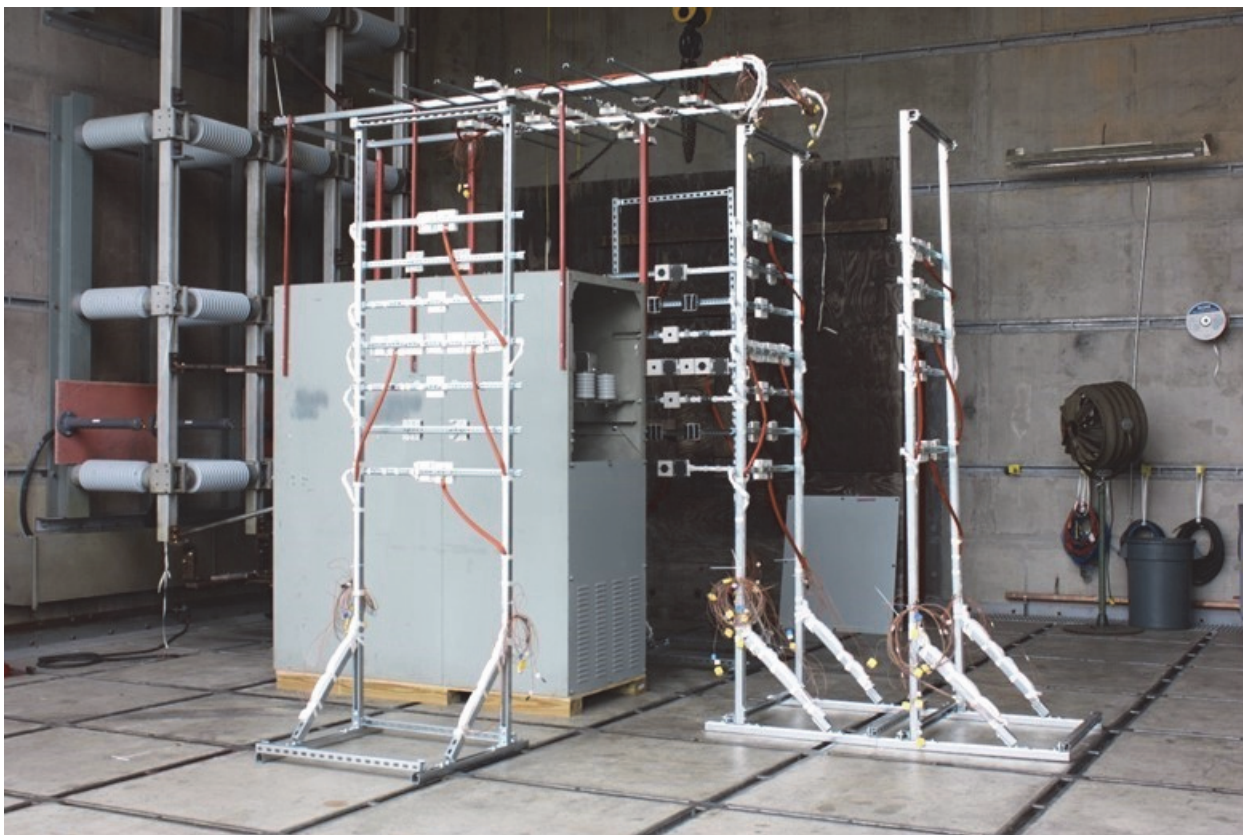
Fig. 35. Photo of Instrumentation Racks during experimental setup.
