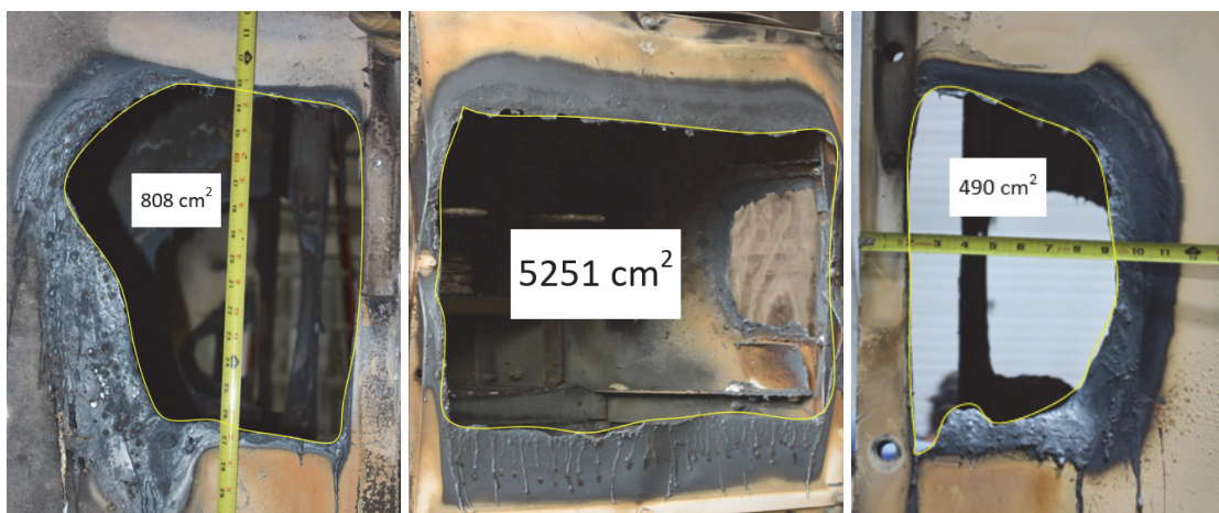
Fig. 51. Photo showing breach opening on far side rear panel (left), upper rear panel (center), and the primary cable compartment bus side upper panel (right). Software used to estimate opening area.
