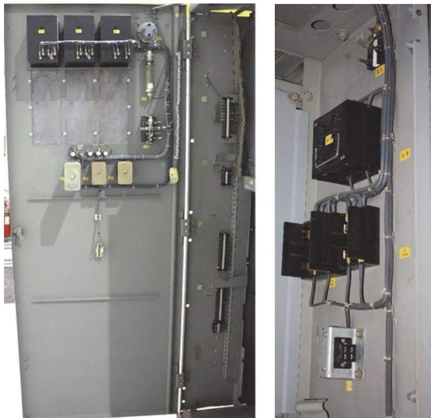
Fig. 9. Photo of combustible component loading in the secondary enclosure
