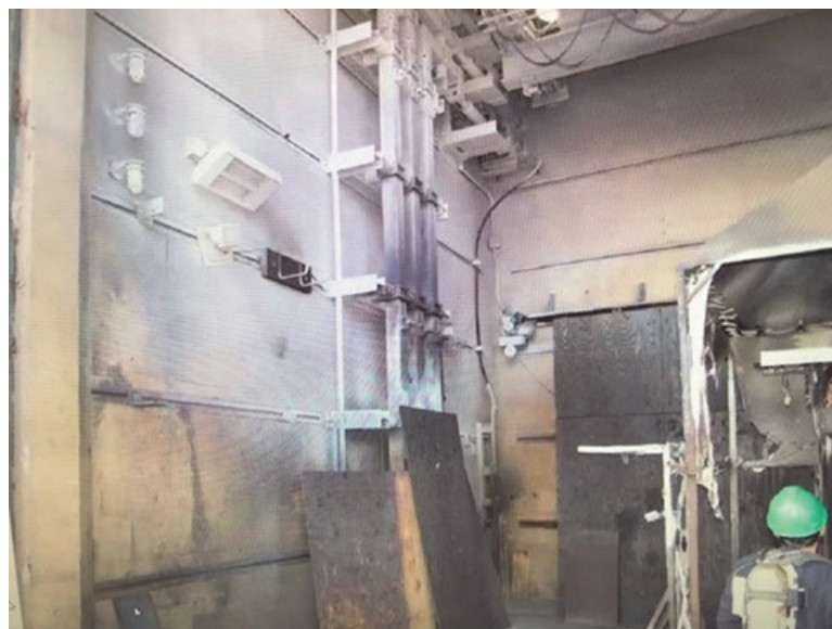
Fig. 58. Conductive white powder residue after previous aluminum bus bar switchgear experiments, which may have consisted of melted Al and evaporated \text{Al}_2\text{O}_3 . (Photo from Phase 1 experiments [6])
