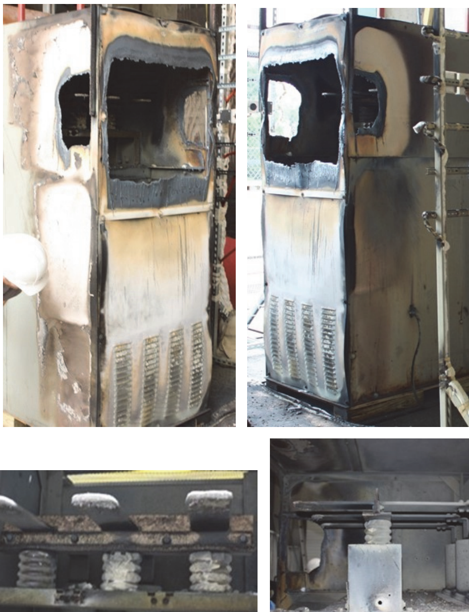
Fig. 48. Enclosure Post-Test 2-21. (Top: back of enclosure; Bottom: remaining bus bar material. Bottom left as viewed from rear of enclosure, bottom right as viewed from the side at the rear of the enclosure with the side panel removed.)
