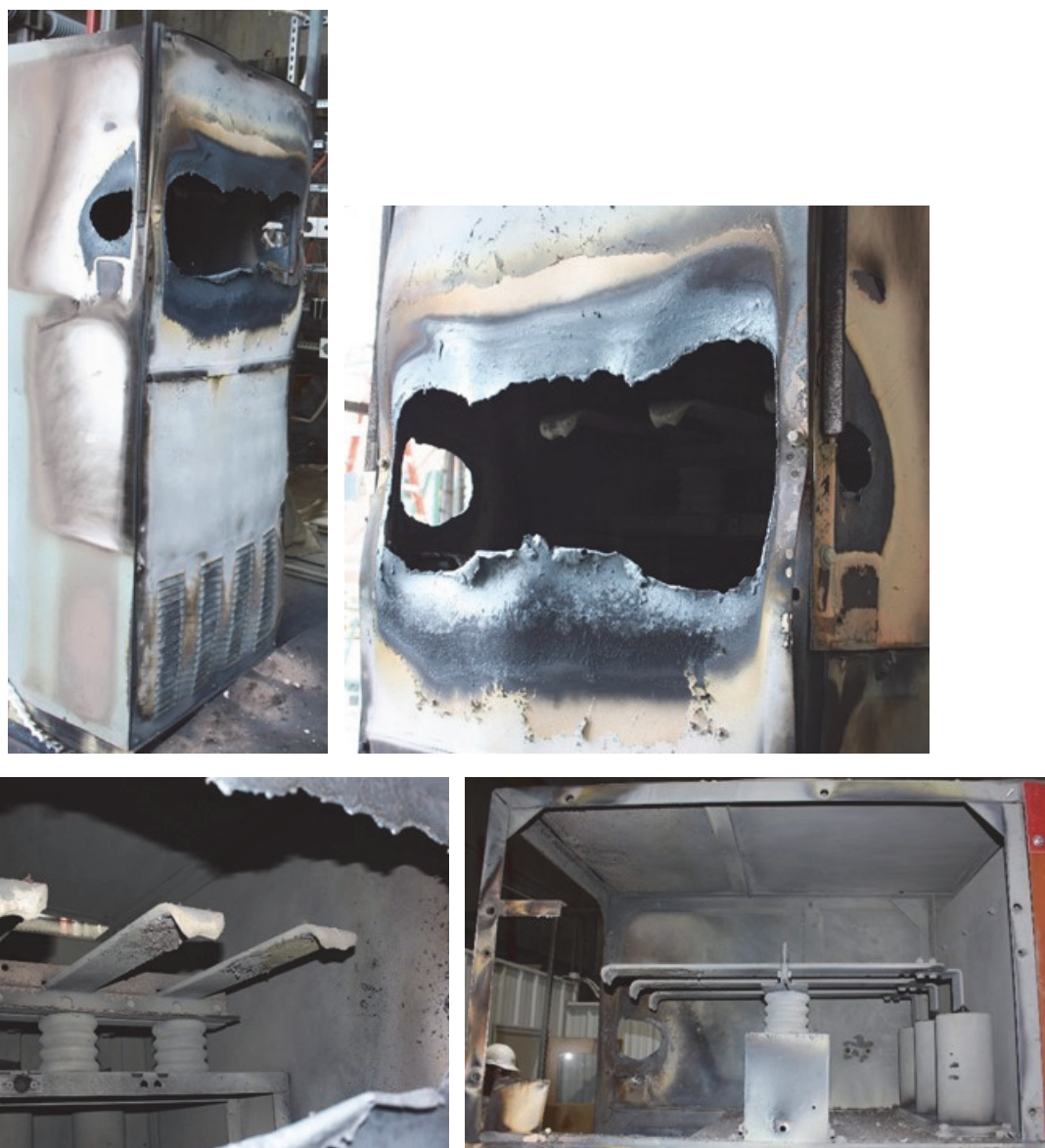
Fig. 69. Enclosure Post-Test 2-22. (Top: back of enclosure; Bottom: remaining bus bar material. Bottom left as viewed from rear of enclosure, bottom right as viewed from the side at the rear of the enclosure with the rear and side panels removed.)
