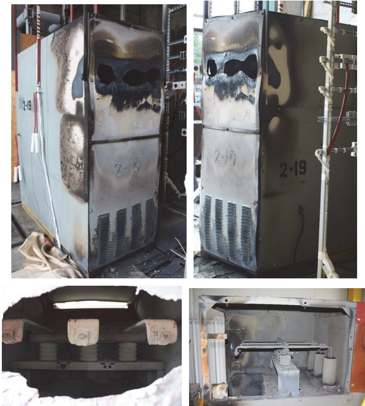
Fig. 38. Enclosure Post-Test 2-19. (Top: back of enclosure; Bottom: remaining bus bar material. Bottom left as viewed from rear of enclosure, bottom right as viewed from the side at the rear of the enclosure with the side panel removed.)
