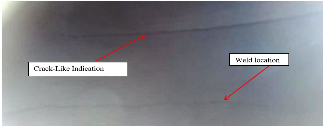
Figure 3 Crack-Like Indication Identified by Visual Inspection
