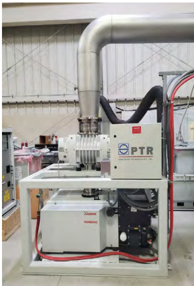
Mechanical pump package
