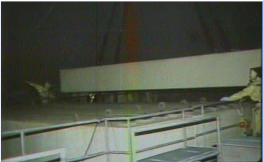
Containment building polar crane load test using 40-ton missile shield blocks that are normally positioned over the reactor vessel service structure.
