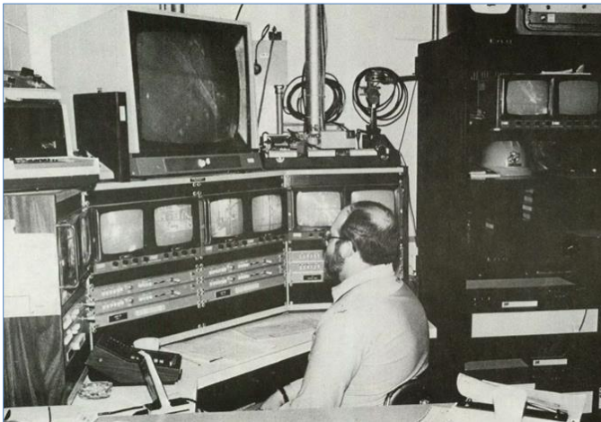
The remote coordination center located in the TMI-2 turbine building contained the control functions for entry into the containment building with positions for safety; radiological engineering; operations; entry coordinator; and command center management. (481.15)
