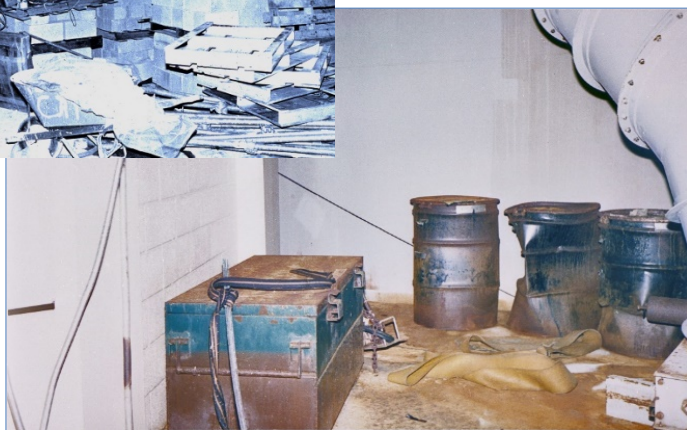
Pre-accident construction-related equipment and materials stored inside the auxiliary building (top) containment building (bottom) became sources of radiation hot spots that complicated decontamination.
