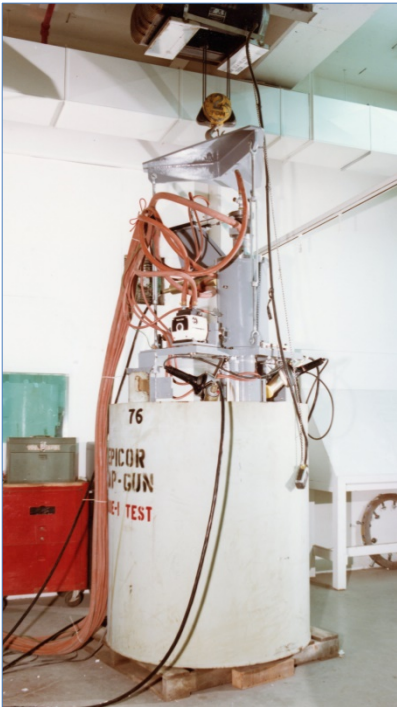
Prototype gas sampler installed on an EPICOR II liner. INEL designed and built the device to sample and vent the liners remotely and to add recombiner catalyst. (481.20)
