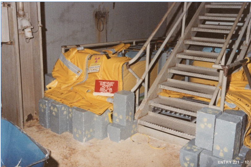
Lead shielding around the enclosed stairwell at the 305-foot elevation (entry level) inside the containment building.
