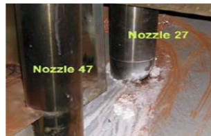
V.C. Summer (Fall 2000): Leaking PWR CRDM Head Penetrations
