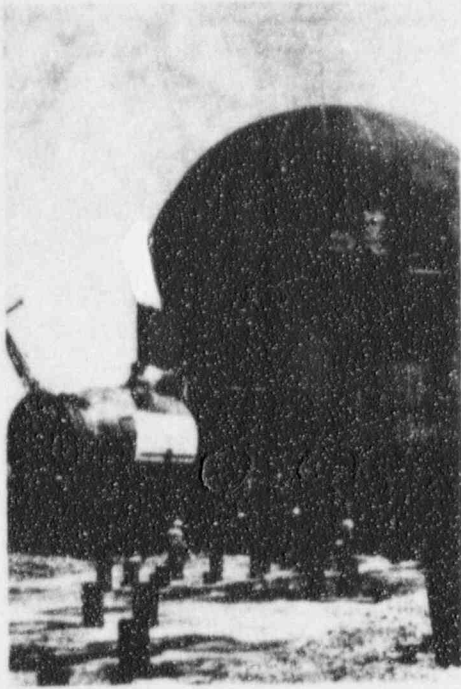
Pressure vessel being moved into PRDC plant, July 1958. (Courtesy of Combustion Engineering, Inc.)
