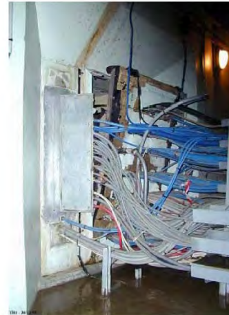
Failure of Cable opening
