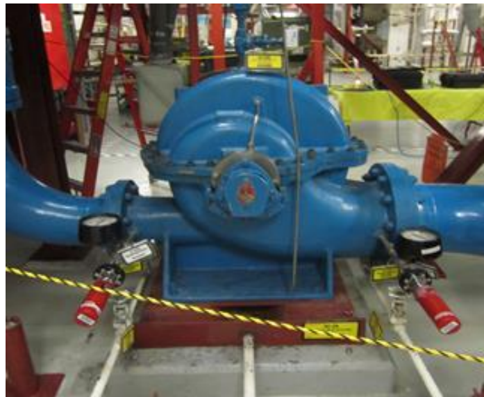
Installation of Pressure Gauges on the CCW “A” Pump to Measure Suction (right), Discharge (left) Pressures (Source: Author)
