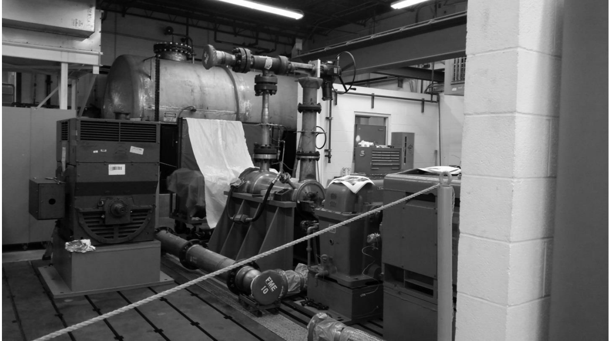
Figure 1. Loop without SIP Showing Tank, SIP Motor, and Centrifugal Charging Pump Casing
