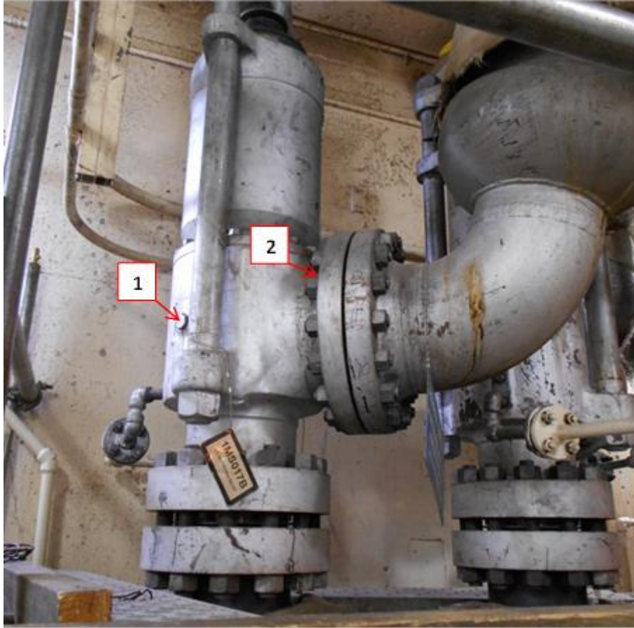
Figure 1. Temperature readings are collected on the valve body (1) and on the tailpipe flange (2).
