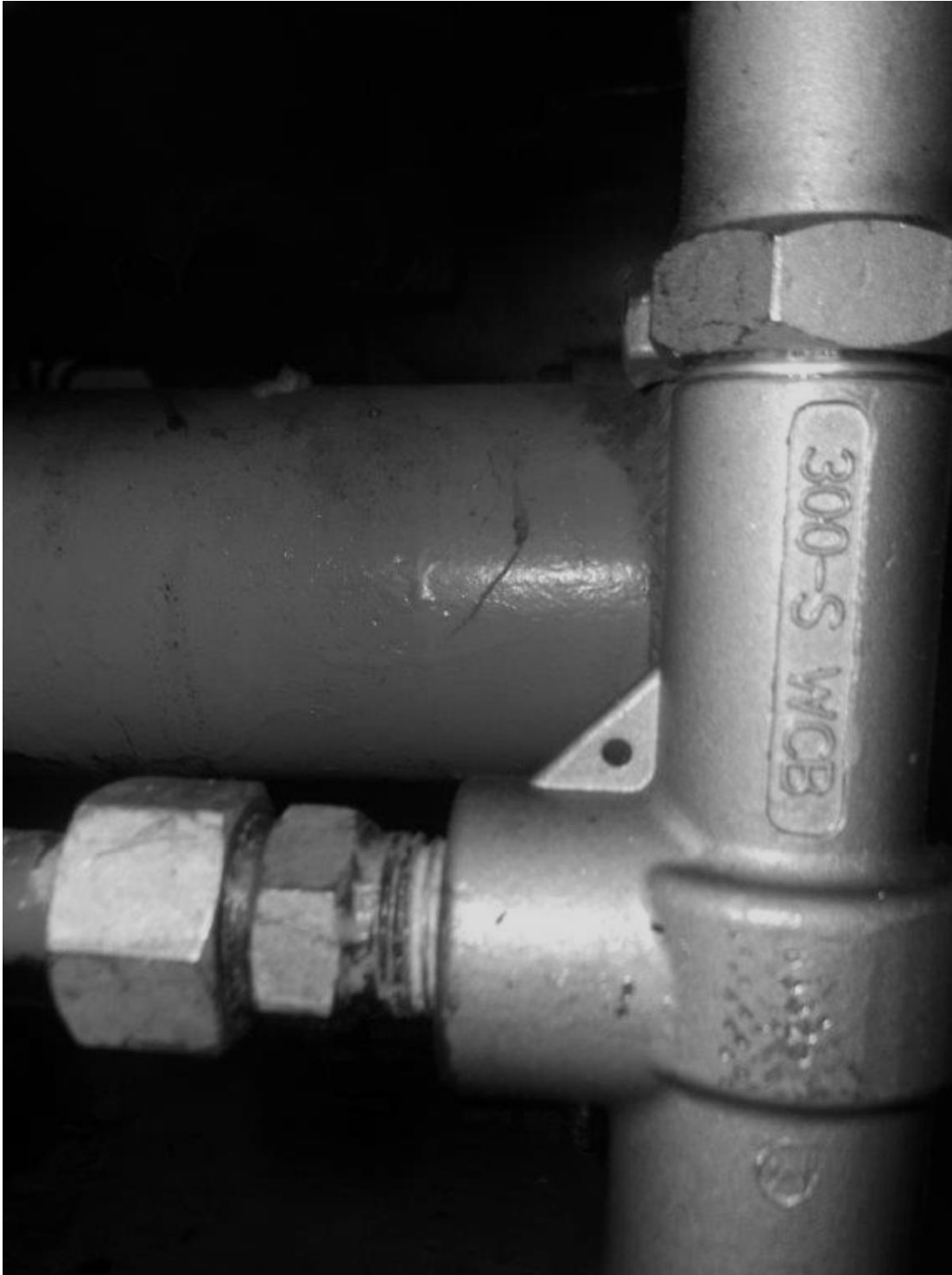
Figure 5. Fulflo PRV Installed at the Pilgrim Station (Source: Author)
