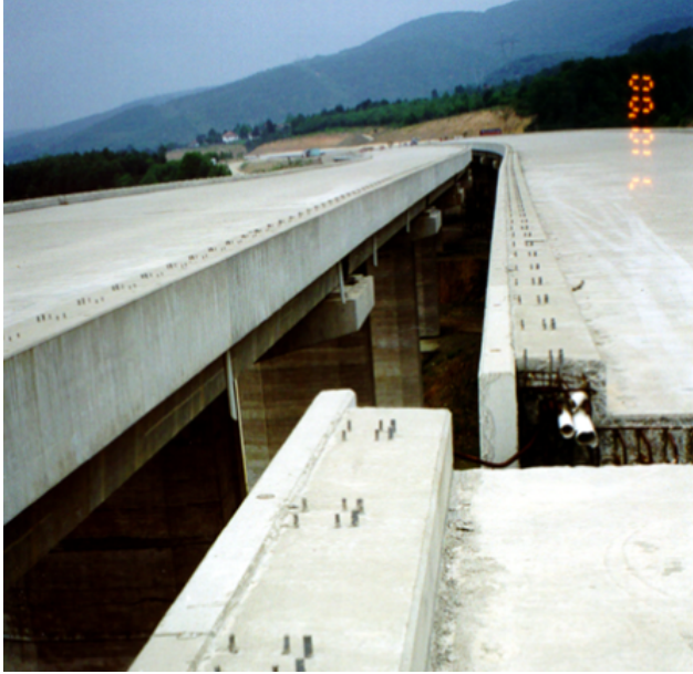
(a) Excessive superstructure movement
