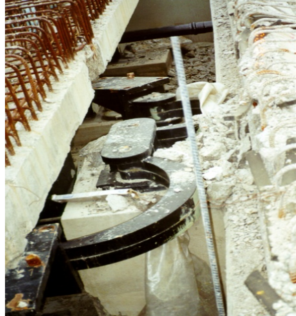
(b) Damaged energy dissipater
