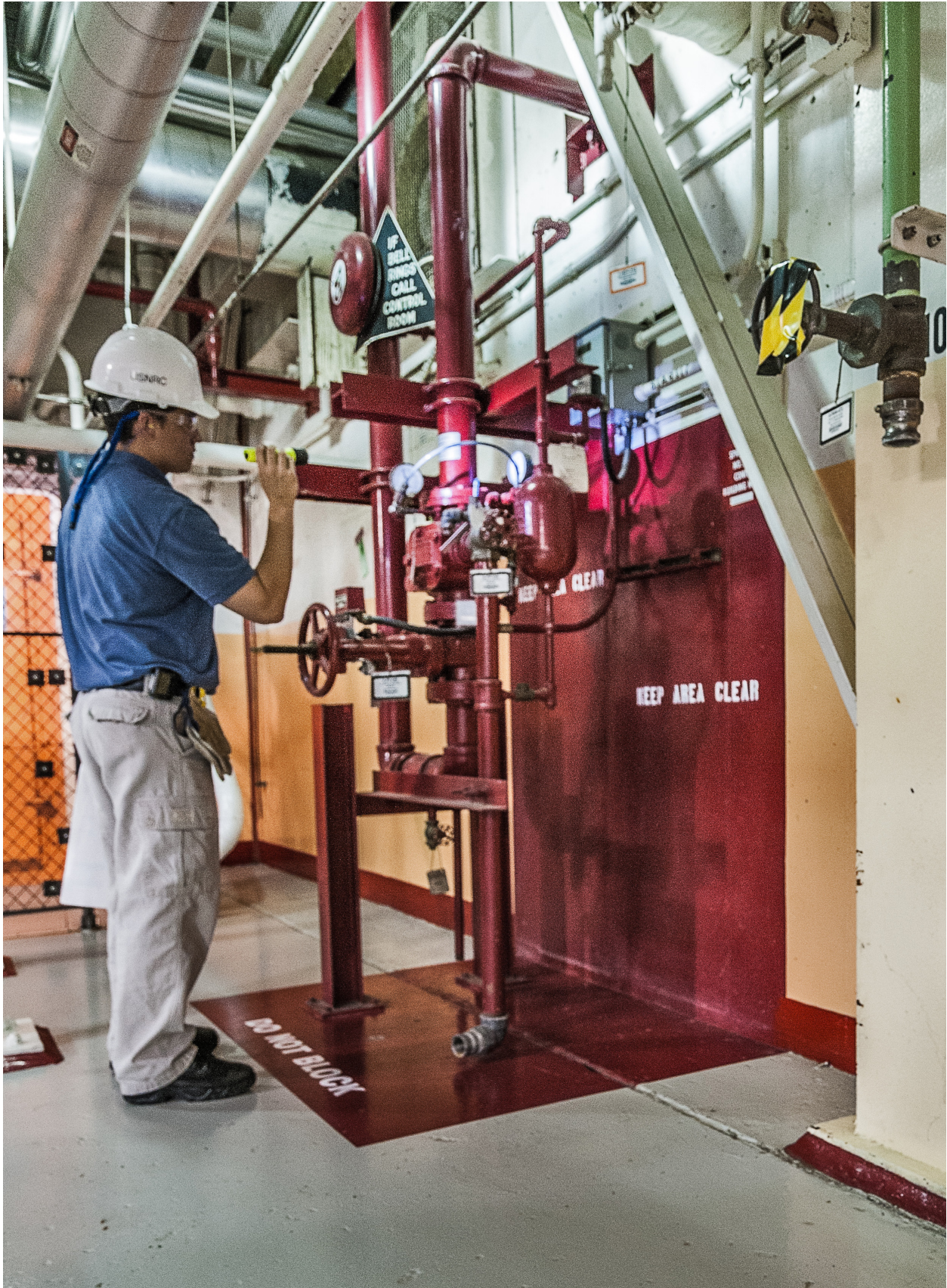
Fire equipment inspection at Calvert Cliffs nuclear power plant.
