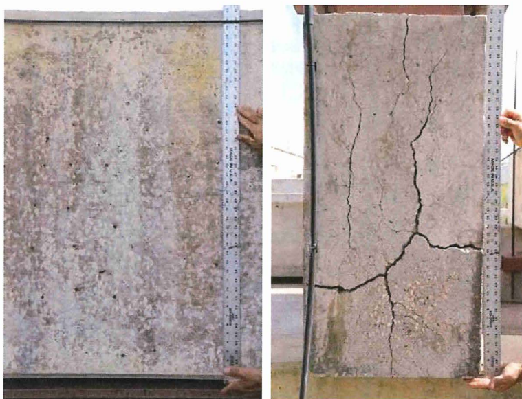
Confined Face of ASR-affected Beam (left); Unconfined face of Same ASR-affected Beam (right)
