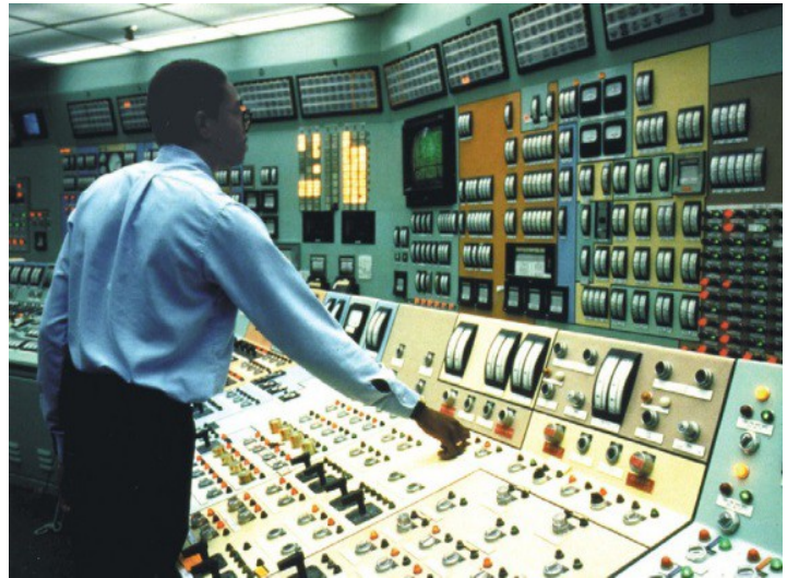
Figure 8.1 Human-System Interface in the Control Room.
