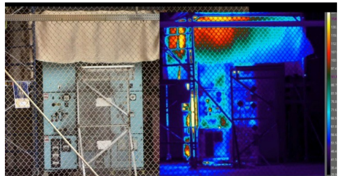
Figure 9.9 High Energy Arc Fault International Test Program – Thermal Camera Imaging.
