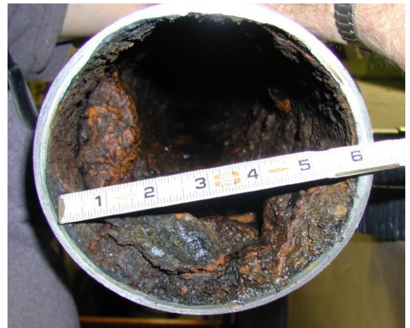
Figure 11.11 Fouling from tubercles in service water system (NRC presentation at NRC/NEI public meeting, Dec 4, 2014, ML14338A376).
