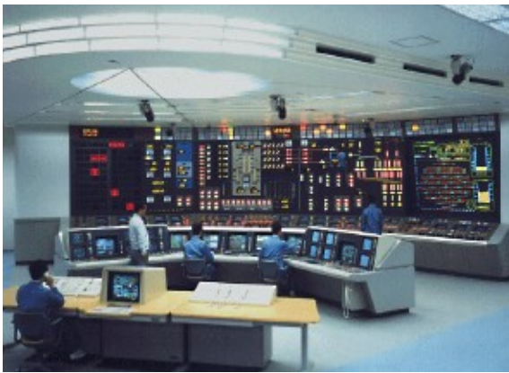
Figure 13.1 Highly Integrated Control Room.
