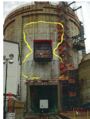
Figure 12.6 Delamination of Crystal River Unit 3 PCCV.
