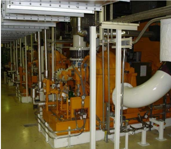
Condensate Booster Pumps
