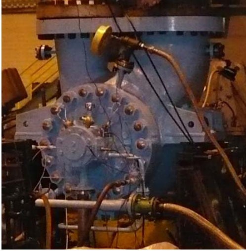
Feed Water Pump
