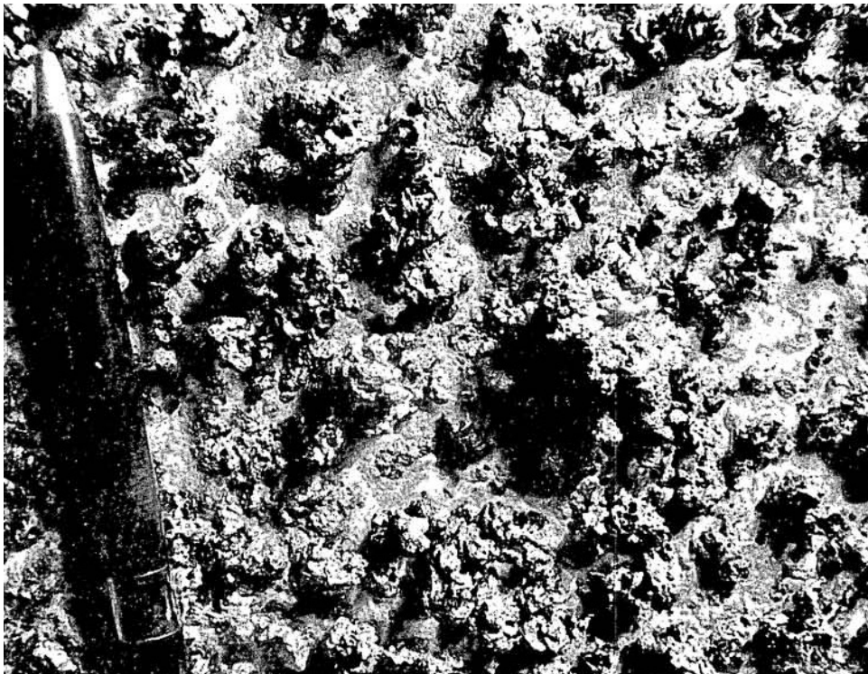
Figure B-10 Close-up of deposits on walls in denitrator room after explosion [McKibben 1976]
