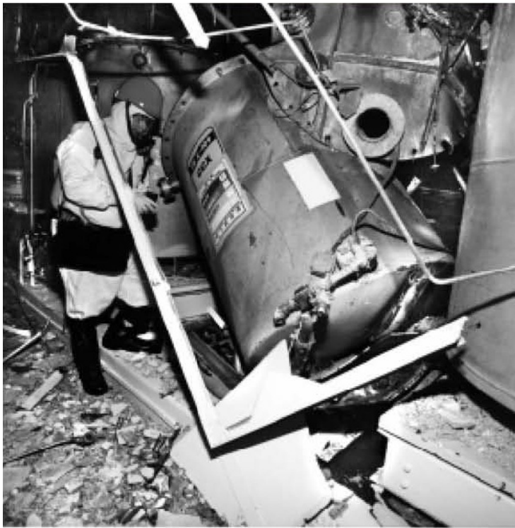
Figure B-22 A post-explosion photo showing the displacement of A-109 Tank [Halow 1998]
