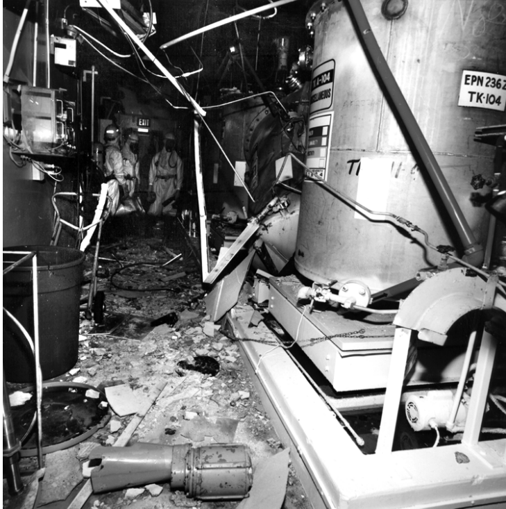
Figure B-21 A post-explosion photo of the tanks inside Room 40 and the location of agitator motor [Harlow 1998]
