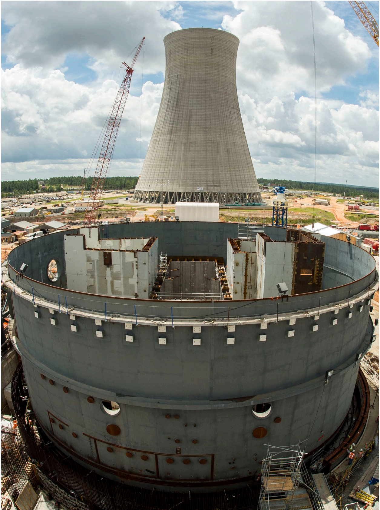
Vogtle Unit 3 nuclear island containment with cooling tower in background. Photo courtesy of Georgia Power
