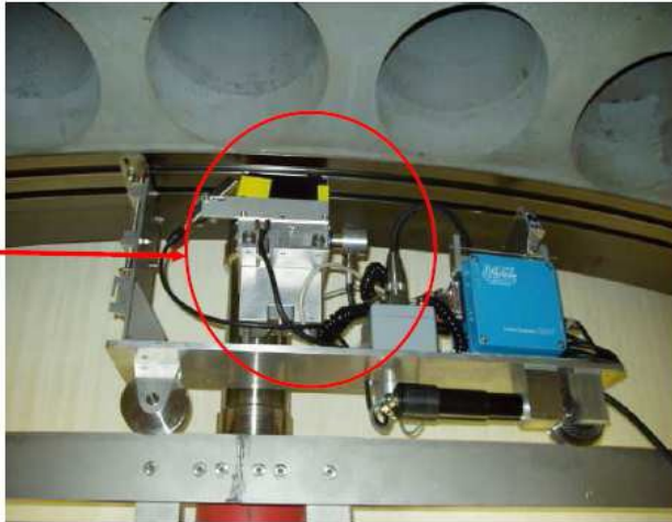
Single Device for Inspection and Laserscan of seal groove surfaces at the RPV closure head
