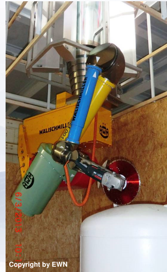
Opening of the Off gas scrubber
