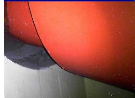
Venting pipes sleeve end
