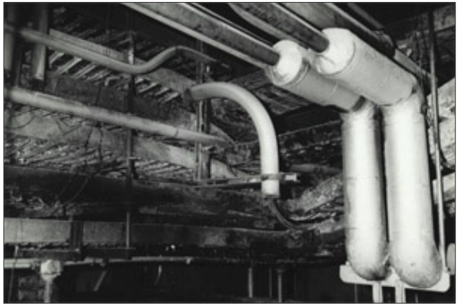
Browns Ferry reactor building after the fire
