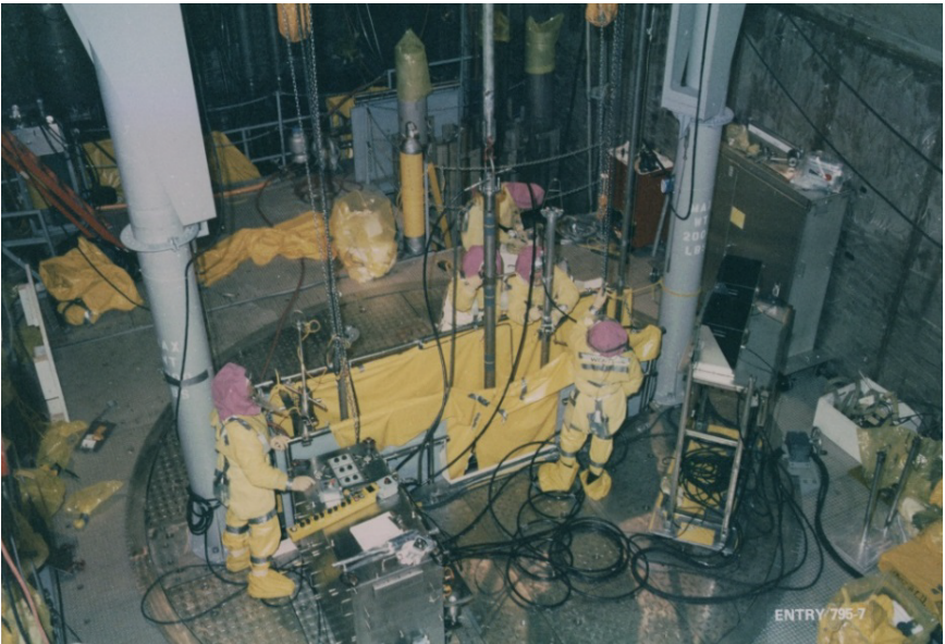
Workers perform defueling operations from a shielded defueling work platform, which was located 9 feet above the reactor vessel flange. The platform had a rotating surface with 6-inch steel plates and a diagonal slit for access into the reactor vessel for removing debris.
