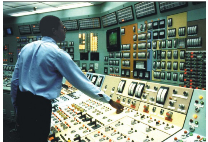
Figure 8.1 Human-System Interface in the Control Room.
