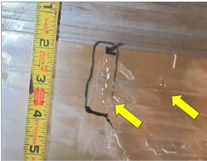
Figure 11.7 Leakage from PWSCC cracks in a steam generator hot leg nozzle.
