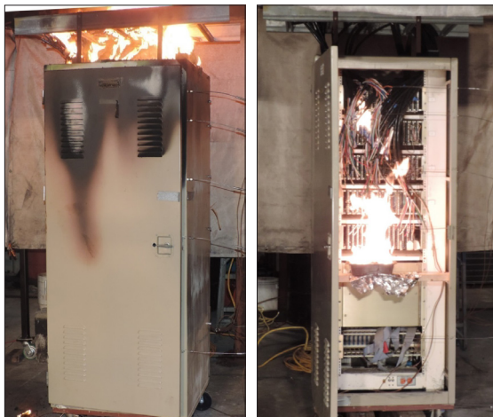
Figures 9.12 and 9.13 Characterizing Heat Release Rates from Electrical Enclosures.
