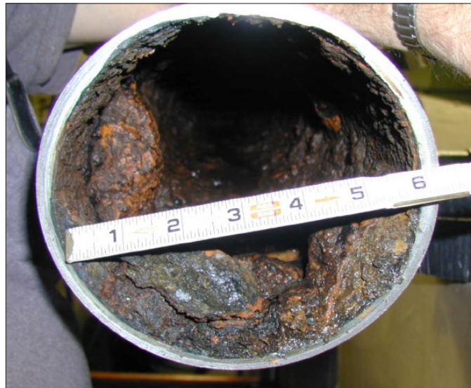
Figure 11.15 Fouling from tubercles in service water system (NRC presentation at NRC/NEI public meeting, Dec 4, 2014, ML14338A376).
