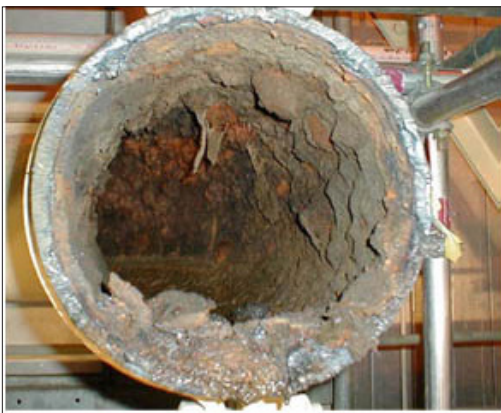
Figure 11.12 Corroded carbon steel pipe.
