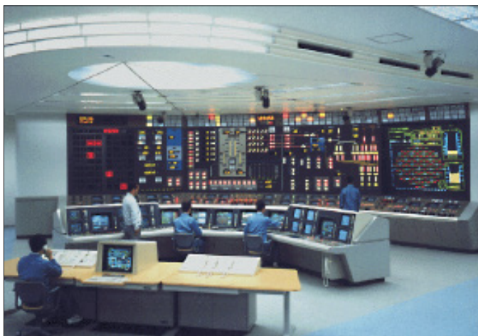
Figure 13.1 Highly Integrated Control Room.
