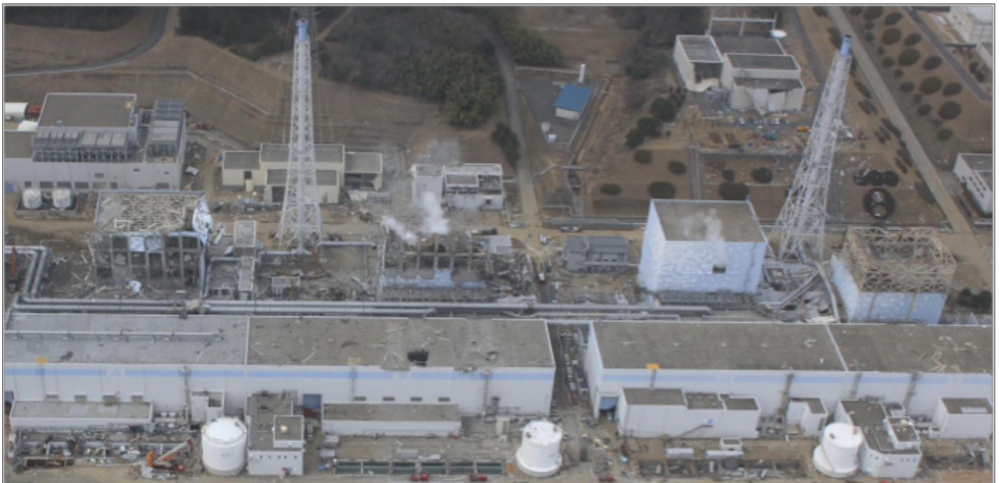
Figure 14.1 Fukushima Units 1, 2, 3, and 4 after the accident showing extensive damage to the reactor buildings.
