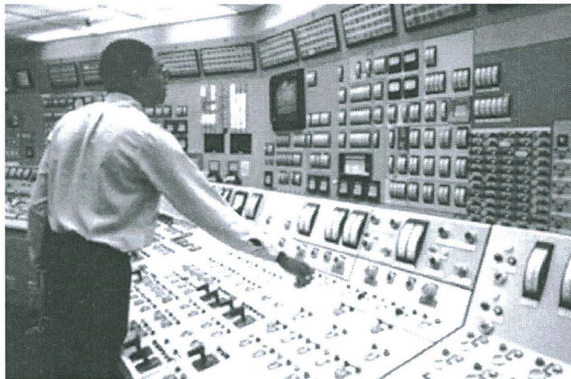
Control Room in a Nuclear Power Plant
