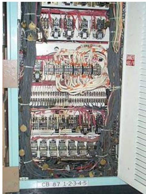
Figure A.3: Example of a Cabinet inside the Main Control Room
