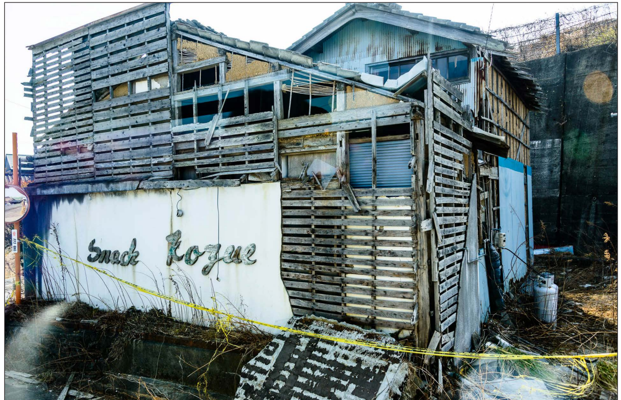
Destroyed store in Tomioka, Fukushima Prefecture, Japan.
