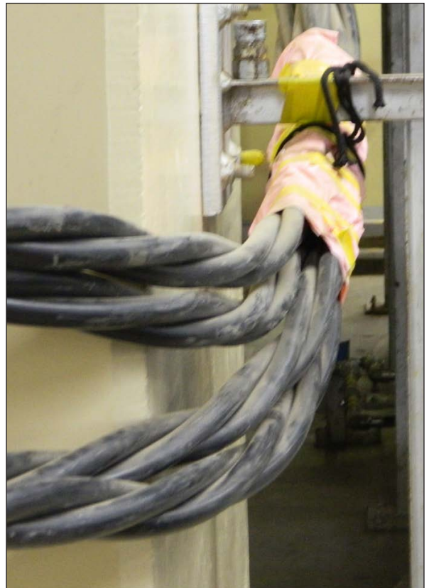
Temporary cables at the Fukushima Daini Nuclear Power Site.
