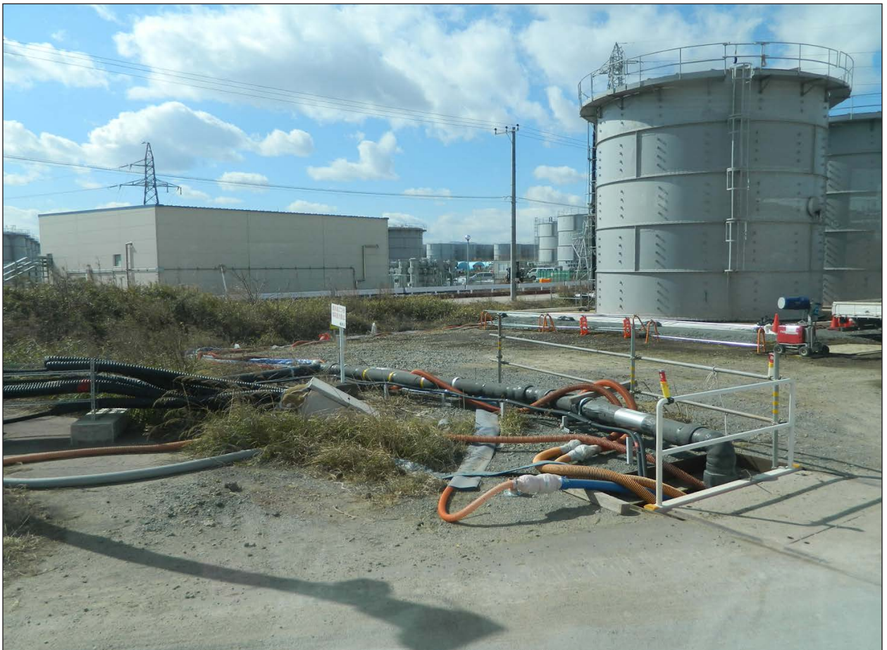
Cables and hoses at the Fukushima Daiichi Nuclear Power Site.
