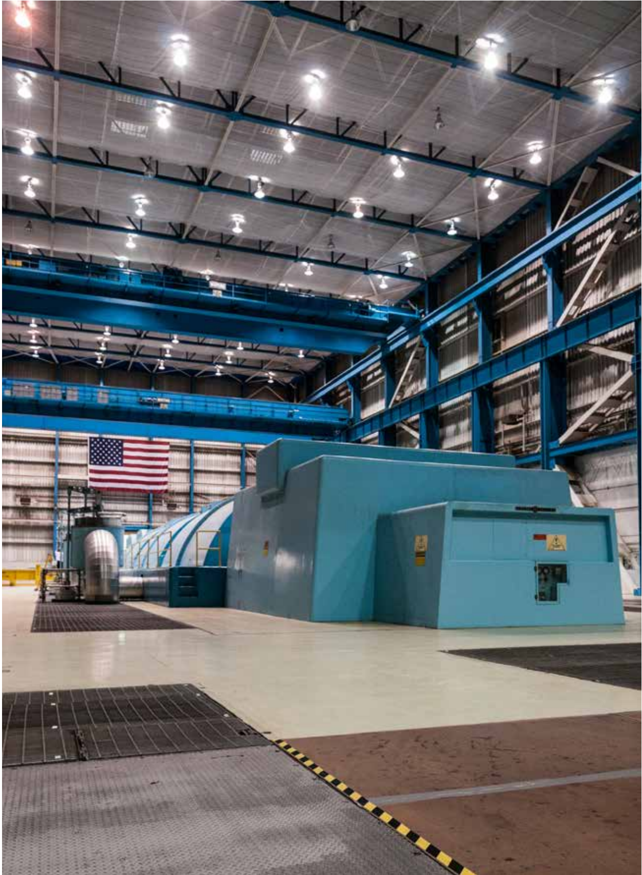
Nuclear steam turbine.
