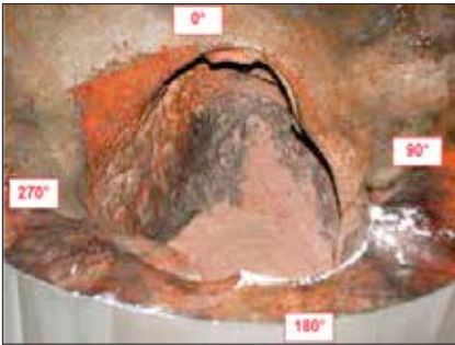
Close-up view of the cavity.
