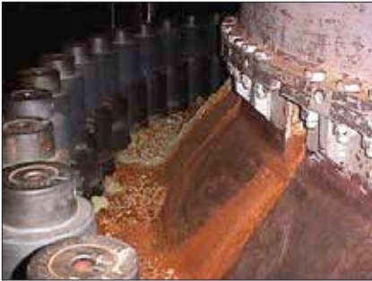
Reactor pressure vessel head flange area showing significant amounts of boric acid deposits (photo taken during the 2000 refueling outage at Davis-Besse Nuclear Power Station).
