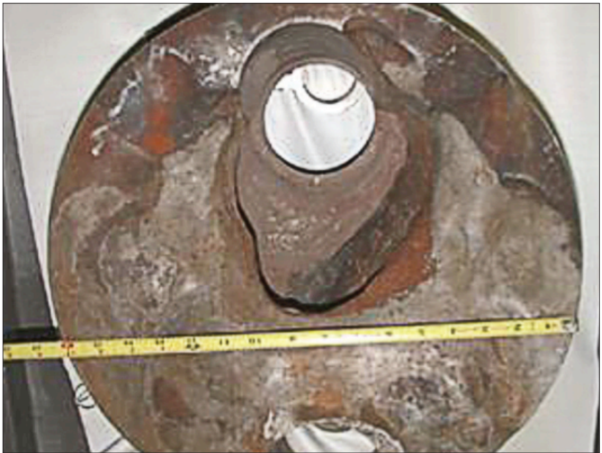
Photo of the cavity after it was removed from the vessel head.
