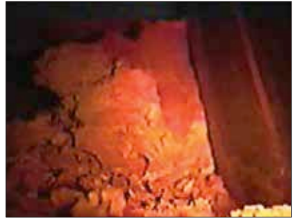
Boric acid deposits accumulating near a CRDM nozzle (still photo of video taken during the 2000 refueling outage at Davis-Besse Nuclear Power Station).
