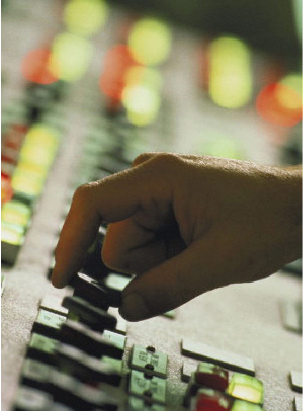
Control panel at a nuclear power plant.
