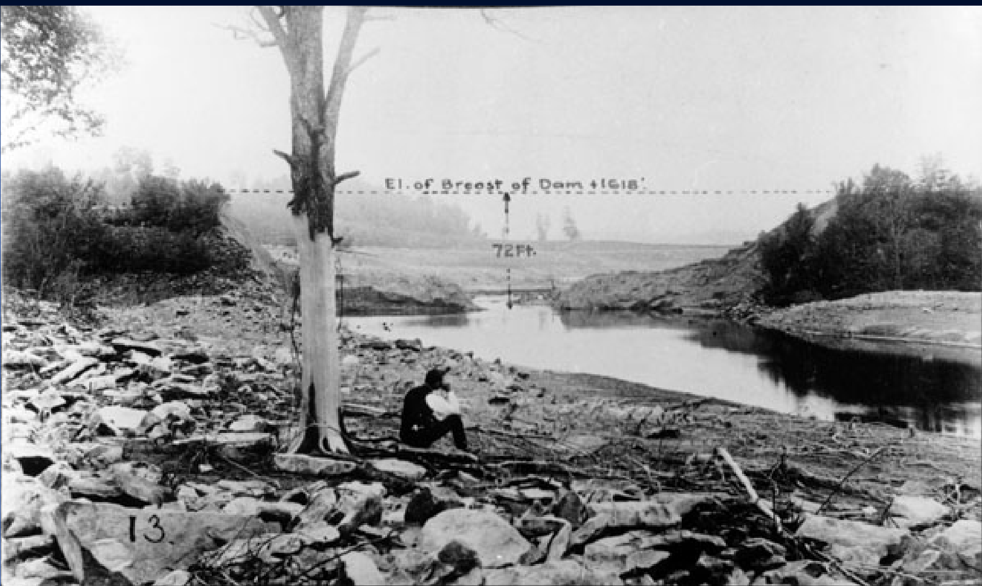
LOOKING EAST THROUGH BREAK IN DAM
