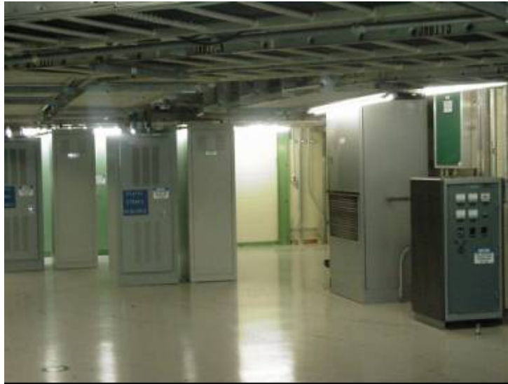
Figure E-2. Photograph of the CSR used for analysis. Note that the cables are located in the trays in the overhead.
