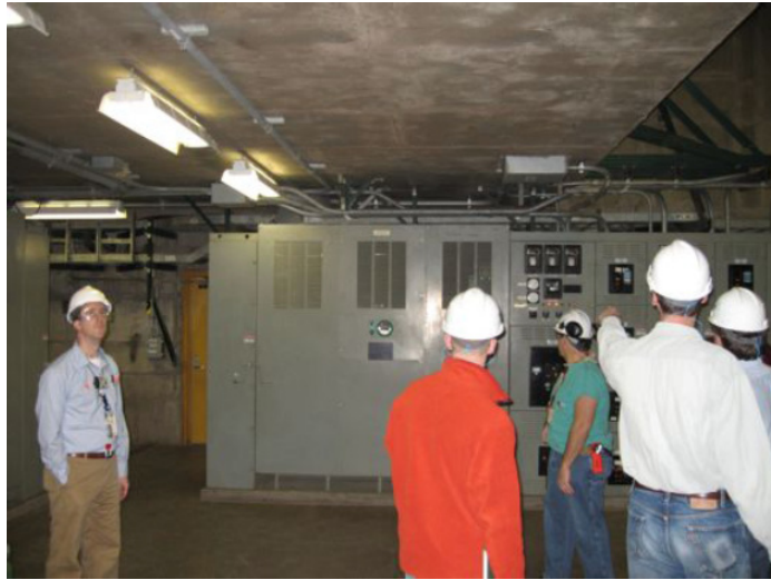
Figure D-2. Typical electrical cabinet in the lower part of the SWGR.
