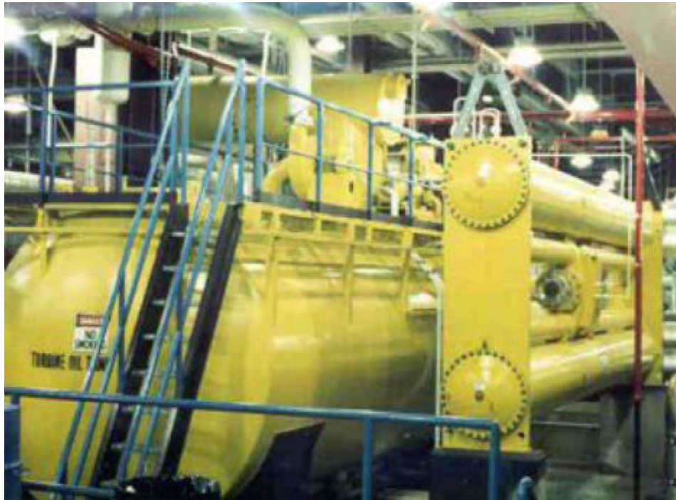
Figure F-2. Main turbine lubricating oil tanks in the turbine building.
