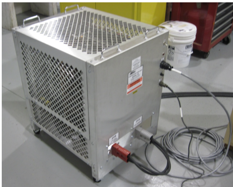
Figure 2-4 600 amp capacity resistive load bank
