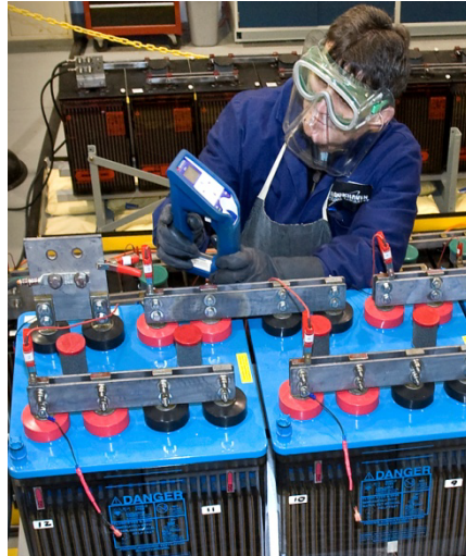
Figure 1-3 Specific gravity readings using a digital hydrometer
