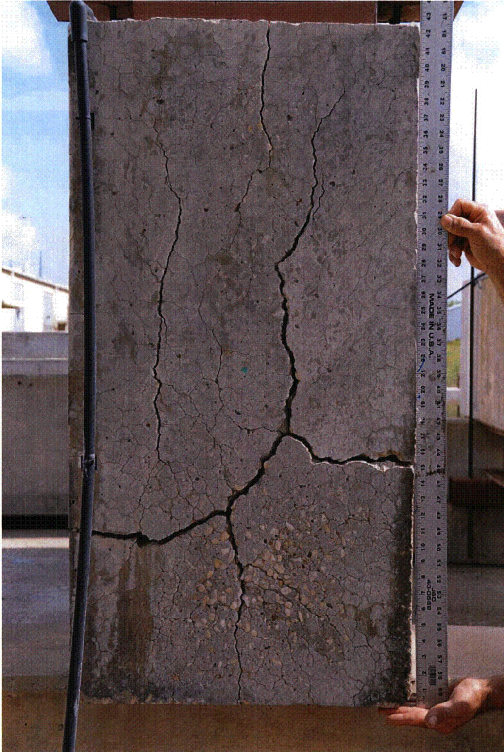
Figure 4-3. End of ASR-Affected Beam (Unconfined Face)
