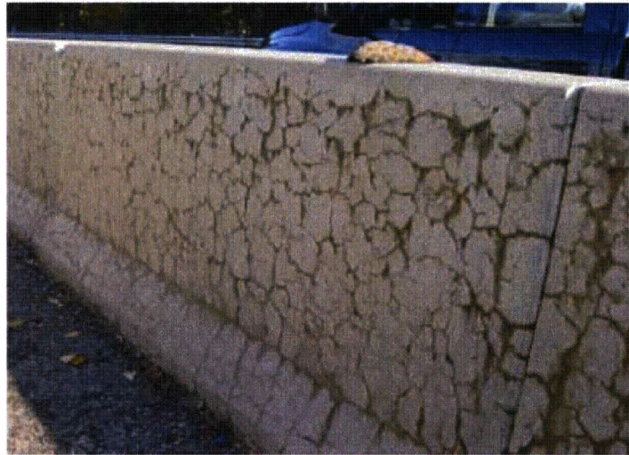
Figure 4-1. Example of ASR Pattern Cracking on Highway Barriers (Reference 9.5.4)
