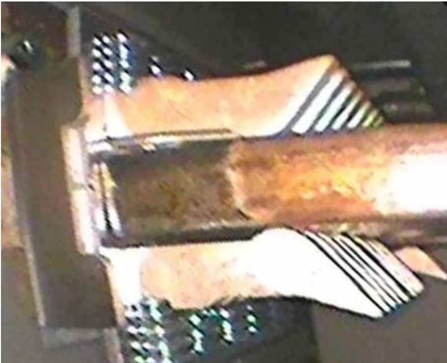
Circuit Breaker Finger & Stab
