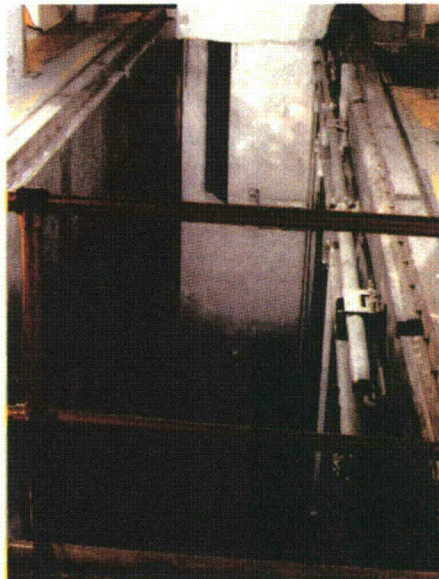
Figure 2-3: Double-lined Spent Fuel Pool
