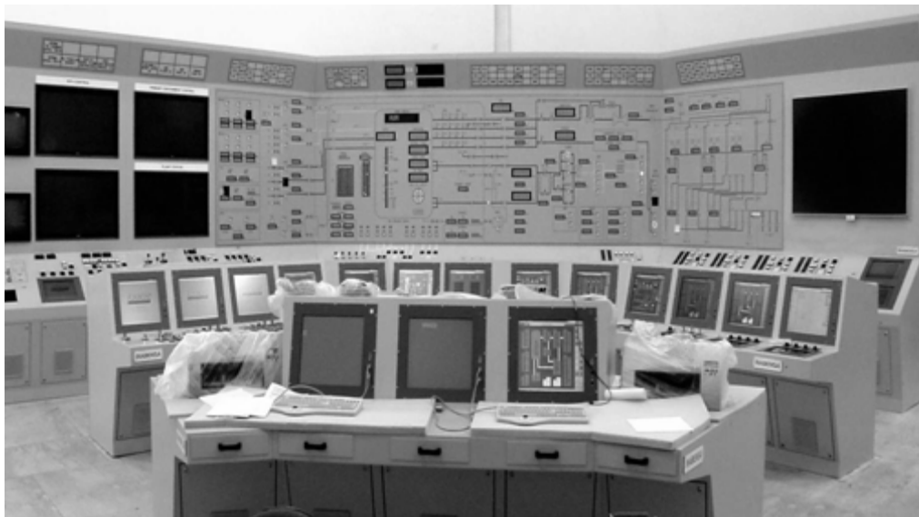
Figure 25. Lungmen plant simulator—a replica of the main control room (Copyright_Feb. 2009 by the American Nuclear Society, La Grange Park, Illinois). 112
