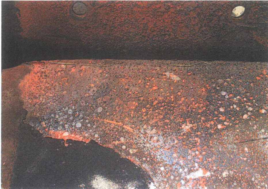
Figure 2-13. Photograph of Plate Girder 9 at the California Department of Transportation Storage Yard. Latex Paint Was Heavily Damaged, Exposing the Red-Colored Lead-Containing Paint.
