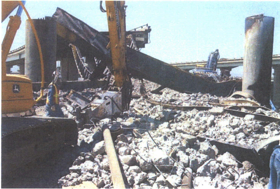
Figure 2-1. Photo During Demolition. Large Hydraulic Hammers Were Used to Break up the Concrete Bridge Deck. The West End of Box Beam Cap 19 Was Still Connected to the Support Column, Whereas the East End Collapsed and Was in Contact With Interstate-880. Picture From California Department of Transportation (2007b).
