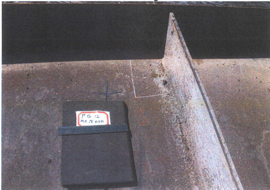
Figure 2-14. Photograph at California Department of Transportation Storage Yard of Plate Girder 12 Near the Bent 18 End. The Latex Paint Was Mostly Intact at This Location.
