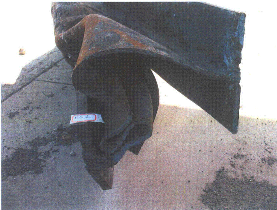
Figure 2-16. Photograph of Plate Girder 1. Buckling of the Plate Girder Appears To Have Occurred at Elevated Temperature.
