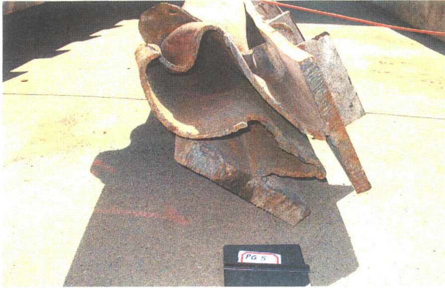
Figure 2-15. Photograph of Plate Girder 5 Believed To Be Between Bent 18 and Bent 19. Buckling of the Plate Girder Appears To Have Occurred at Elevated Temperature.
