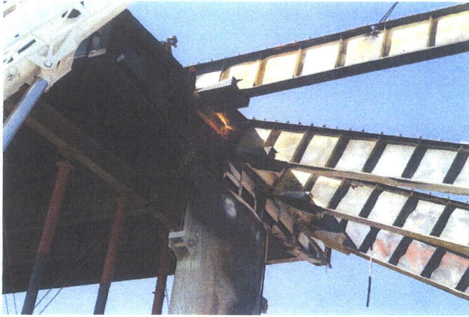
Figure 2-5. Torch Cutting of Plate Girders at Bent 18. Picture From California Department of Transportation (2007c).
