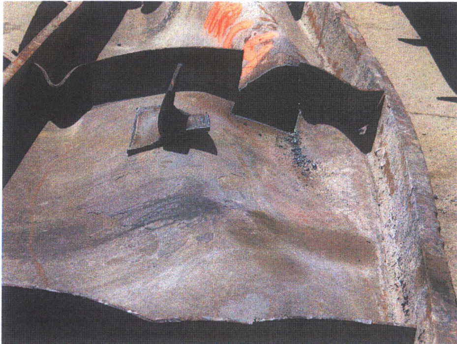
Figure 2-20. Photograph of Plate Girder 5 and Sample NRC 4
