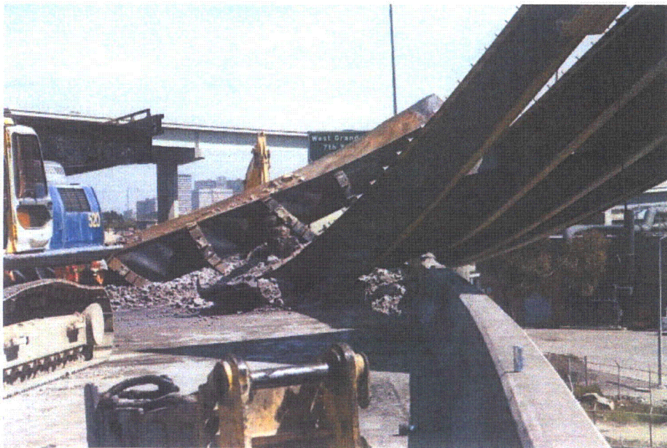
Figure 2-2. Photo During Demolition. View of Plate Girders and Box Beam Cap at Bent 19. Picture From California Department of Transportation (2007c).
