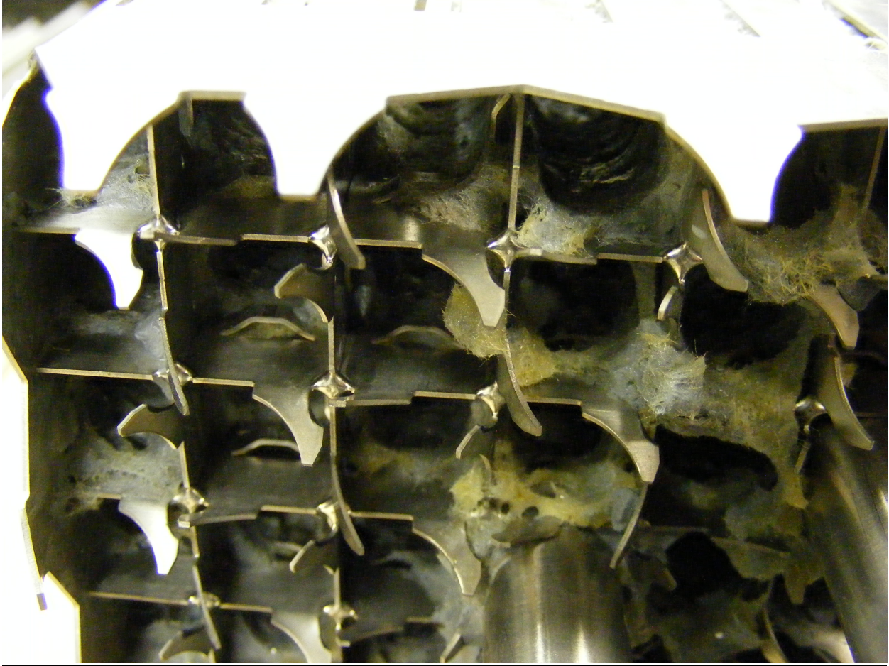
Figure 3: Close-Up View of Debris Deposited at Mixing Grid
