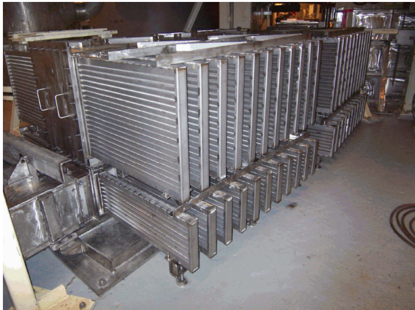
Figure 3: A Section of North Anna's Containment Sump Strainers
