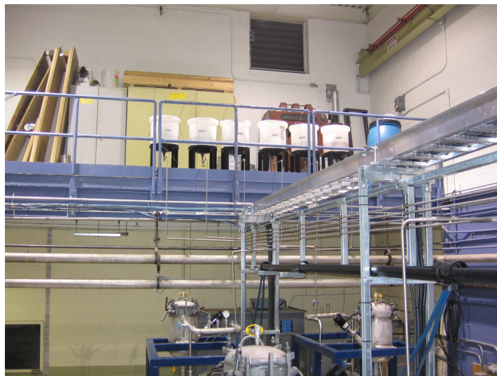
Figure 7: Multi-Loop Rig Head Tank Arrangement
