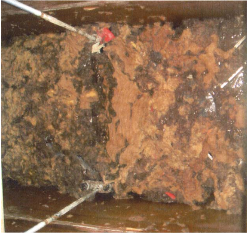
Figure 3. Buoyant Fibrous Debris Located Above Strainer Modules
